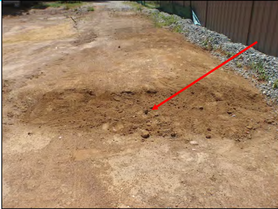
Photograph 3: Northern section of 37 Rich St block after removal of asbestos containing sheet debris from the soil mound
