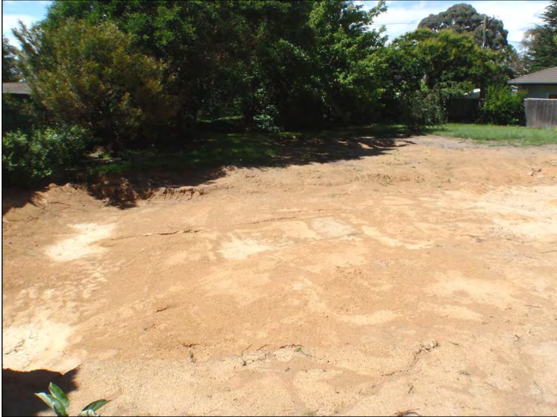
Photograph 3: 56 Belconnen Way Page block after removal of asbestos containing sheet debris scattered in various locations across the top of the soil
