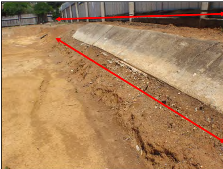
Photograph 2: Southern boundary fence line of the 37 Rich St block after removal of asbestos containing sheet form work and debris – also ACM debris removed from areas at base of incline
