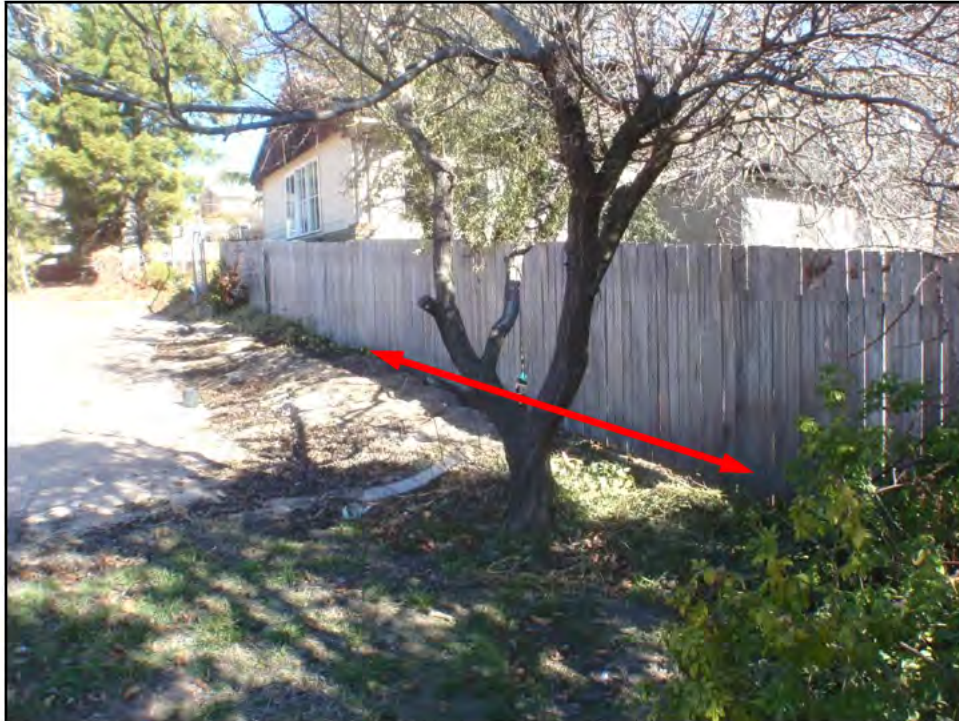
Photograph 1: Western boundary fence line of the 18 Darke Street Torrens block from where asbestos containing sheet was removed from the base of the timber fence
