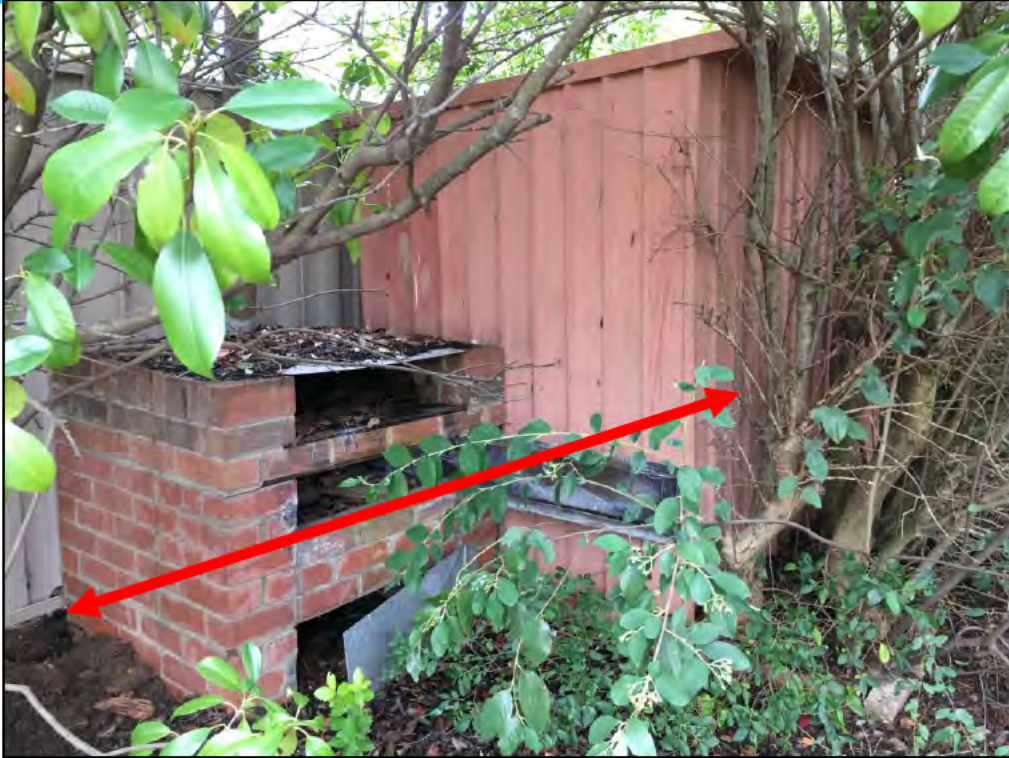
Brick outdoor oven and metal clad shed behind which loose and partially buried asbestos cement sheet debris may remain
