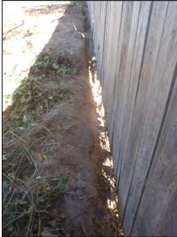
Photograph 3: Western boundary fence line of the 18 Darke Street Torrens block after removal of asbestos containing sheet from the base of the timber fence
