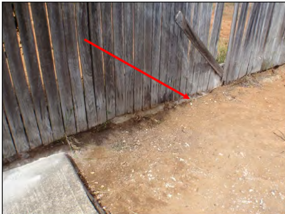
Photograph 6: asbestos containing sheet material remaining along the base of the eastern side boundary fence line adjoining block 29 Rivett St – sheet physically located on 29 Rivett St side of boundary fence and not on the 27 Rivett St block side
