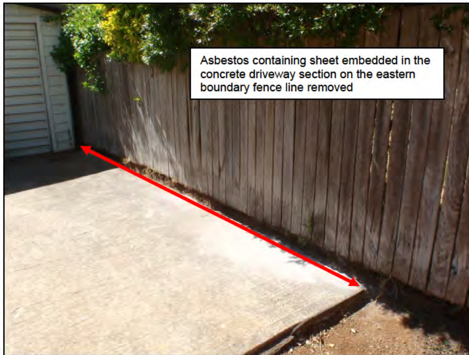
Photograph 1: Location from which asbestos containing sheet embedded in the edge of the concrete driveway section on the eastern boundary fence line was removed
