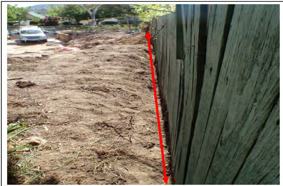
Photograph 2: Removal of non friable asbestos sheeting buried in the garden beds and along the southern boundary fence.
