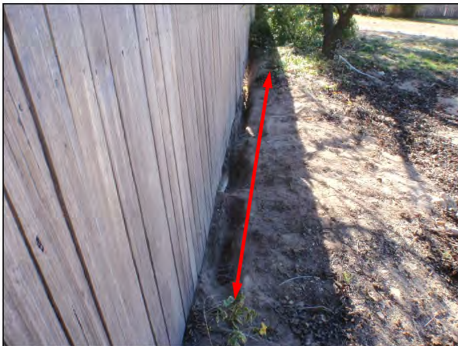
Photograph 2: Western boundary fence line of the 18 Darke Street Torrens block after removal of asbestos containing sheet from the base of the timber fence
