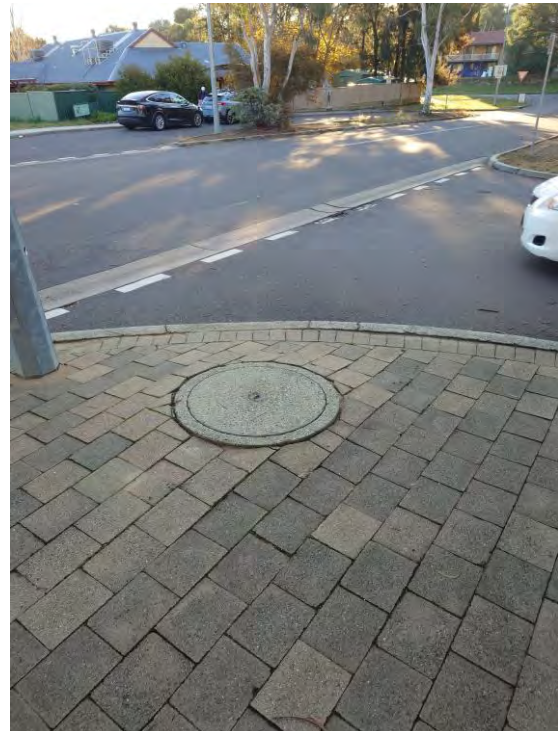
Figure 16 – Sewer Manhole in Georgina Crescent (west) at Intersection with Northern Internal Road
