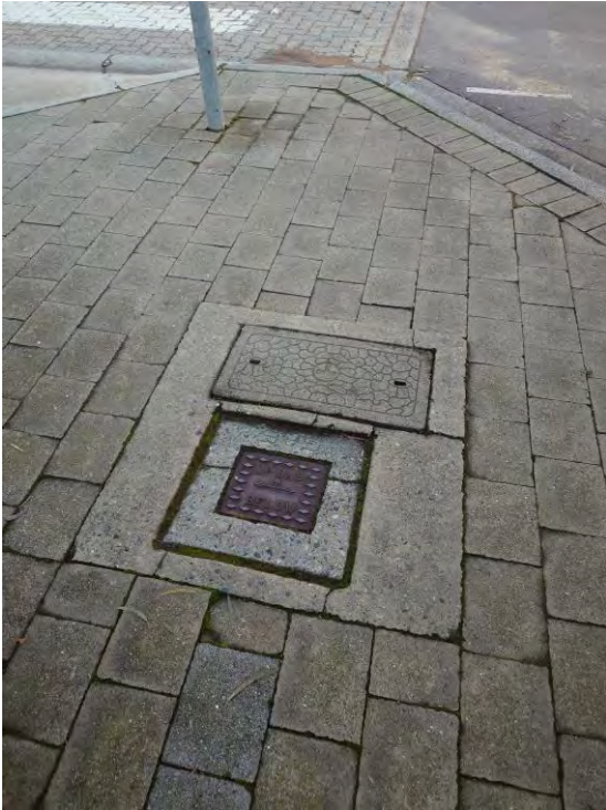
Figure 43 – Gas Marker in the Southern Internal Access Road
