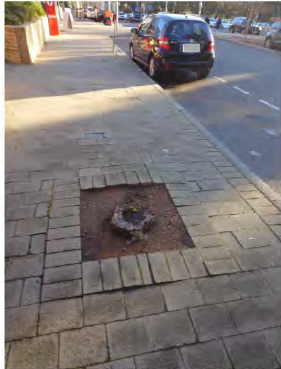
Figure 109 – Tree Stump in Northern Access Road
