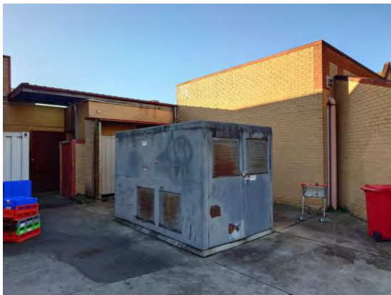
Figure 52 – Electrical Substation S 4565 Near Block 10 Section 88
