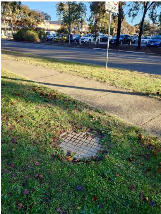
Figure 12 – Receiving Sewer Manhole on DN225 Main in Maribyrnong Avenue
