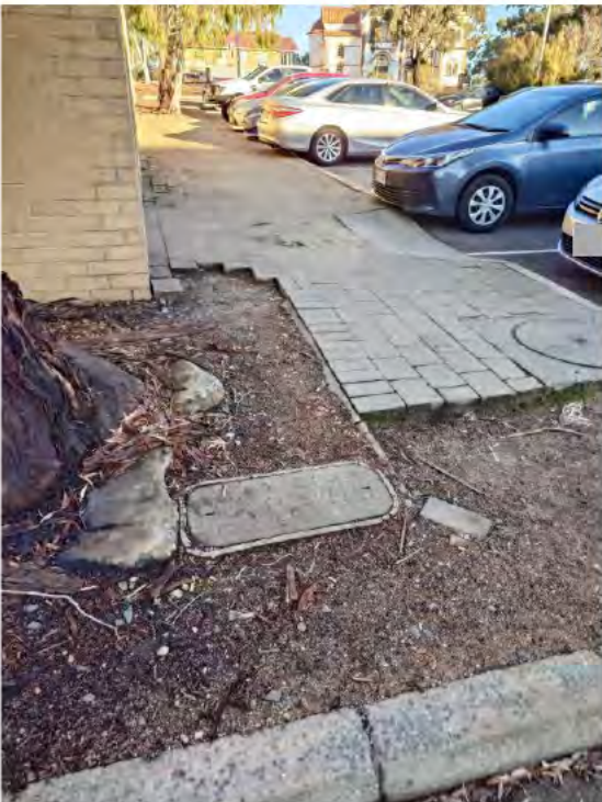
Figure 37 – Telstra Pit Near Block 13 Section 88
