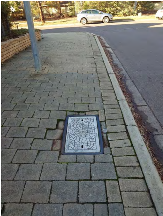
Figure 38 – Telstra Pit in Southern Access Road Near Georgina Crescent (east)
