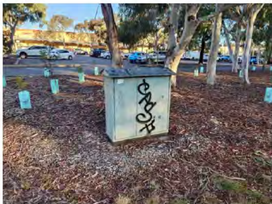
Figure 49 – Electrical Service Point in Southern Verge of Maribyrnong Avenue
