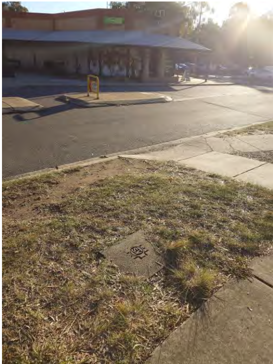
Figure 22 – Stop Valve in Georgina Crescent (east)
