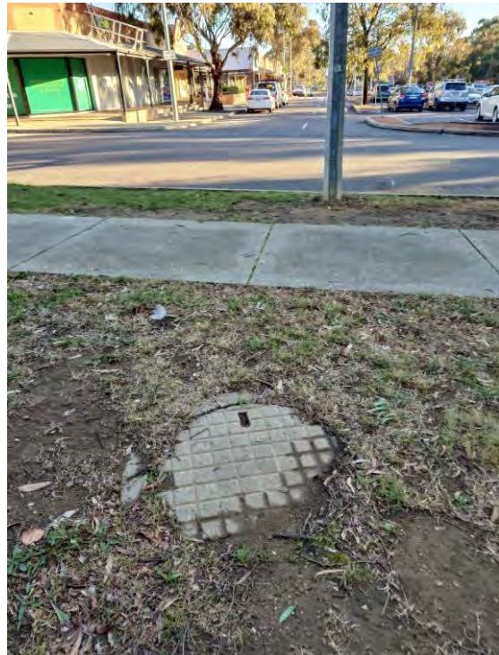
Figure 13 – Sewer Manhole in Georgina Crescent (east) at Intersection with Northern Internal Road
