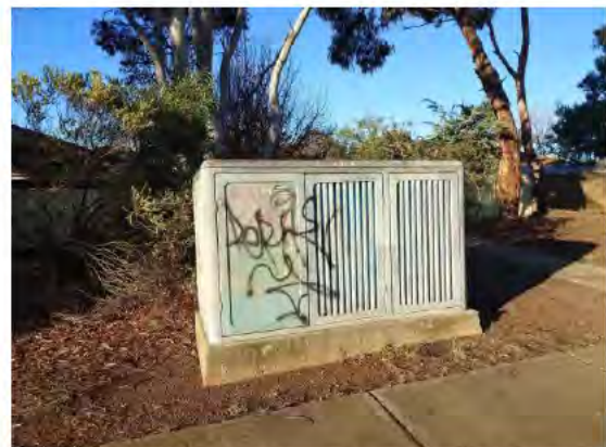
Figure 50 – Electrical Substation S 4057 in East Verge of Georgina Crescent (east)
