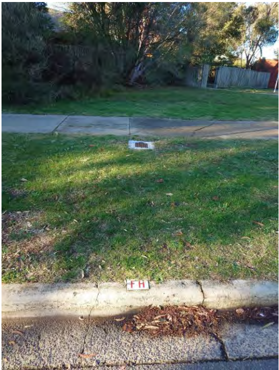
Figure 21 – Fire Hydrant in Georgina Crescent (east)
