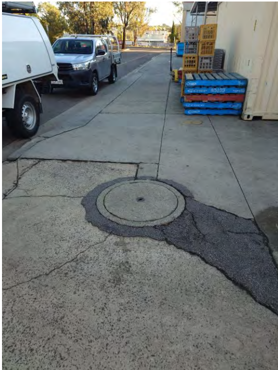
Figure 15 – Sewer Manhole in Southern Internal Road
