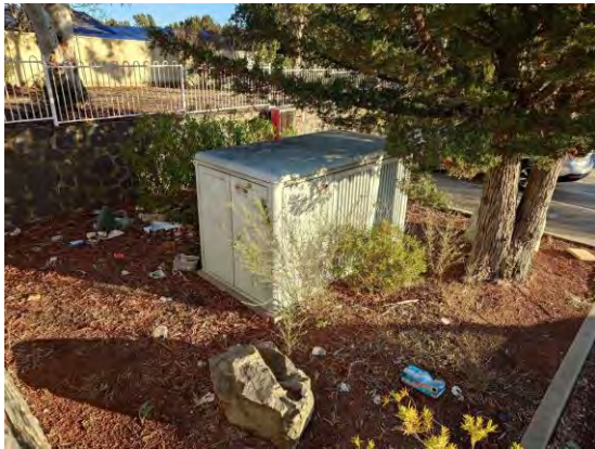
Figure 51 – Electrical Substation S 4895 in Block 4 Section 89 Kaleen
