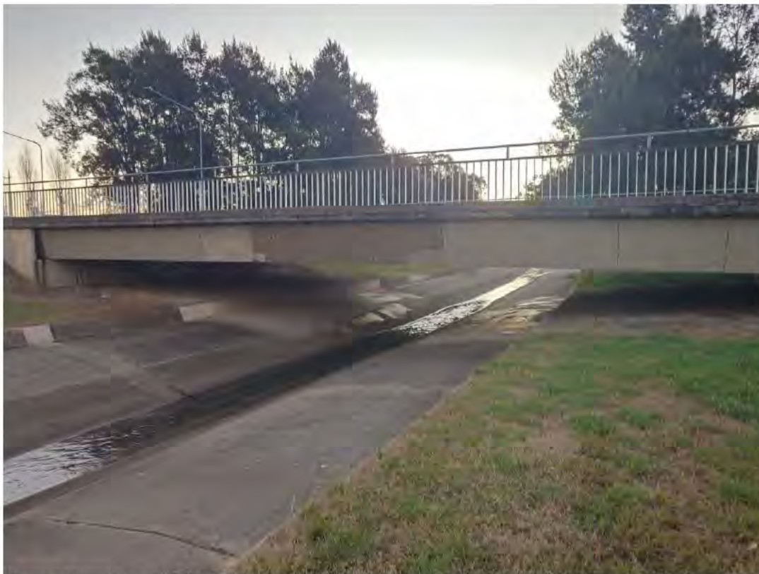
Figure 31 – Concrete Lined Channel in Baldwin Drive and Bridge over Maribyrnong Avenue Looking North
