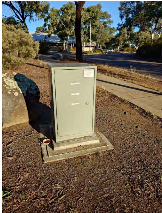
Figure 53 – Streetlighting Control Cubicle in Georgina Crescent (east) East Verge
