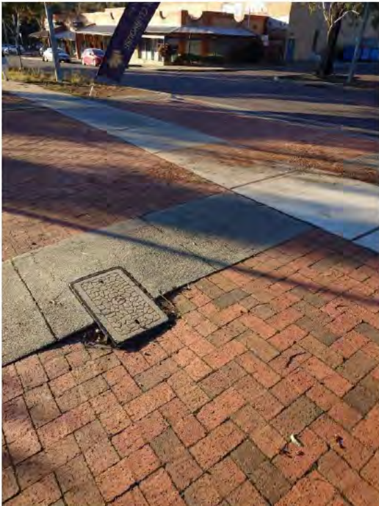
Figure 35 – Telstra Pit in West Verge of Georgina Crescent (west)
