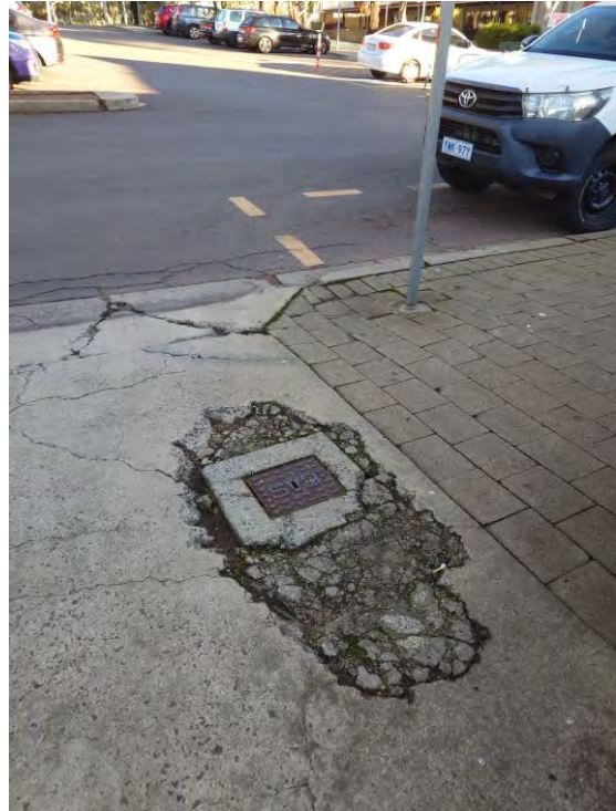
Figure 44 – Gas Isolation Valve in the Southern Internal Access Road
