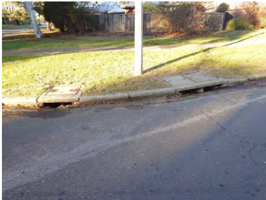
Figure 28 – Stormwater Kerb Side Sumps at Intersection of Georgina Crescent (east) and Maribyrnong Avenue
