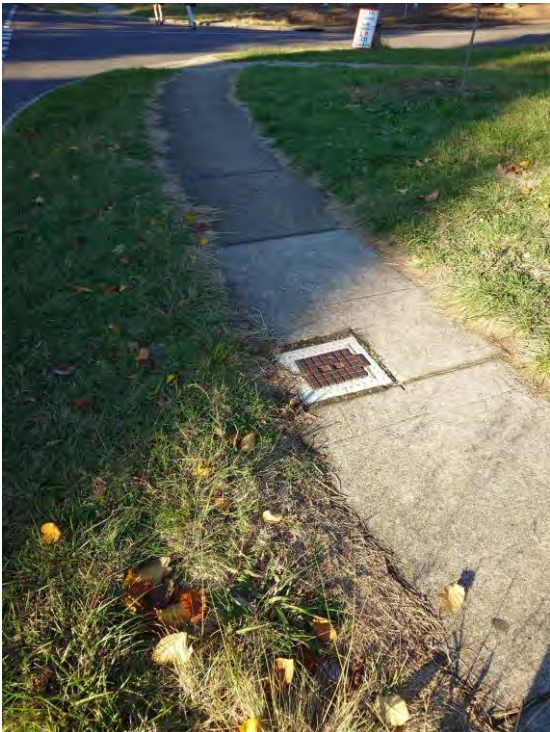
Figure 19 – Fire Hydrant at Intersection of Maribyrnong Avenue and Georgina Crescent (west)
