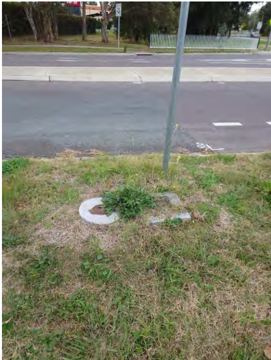
Figure 34 – Existing Fire Hydrant and Stop Valve on DN300 Main in Lhotsky Street
