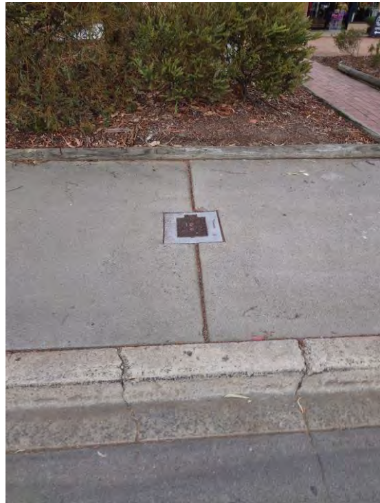
Figure 42 – Existing Fire Hydrant Existing Fire Hydrant in Central Carpark (east)
