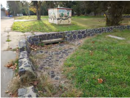
Figure 46 – Existing Stormwater Plantation Sump North of Subject Site
