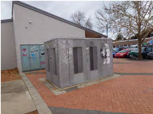
Figure 94 – Electrical Substation S 2721 in Charnwood Place (east)
