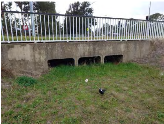
Figure 50 – Stormwater Box Culverts Under Lhotsky Street
