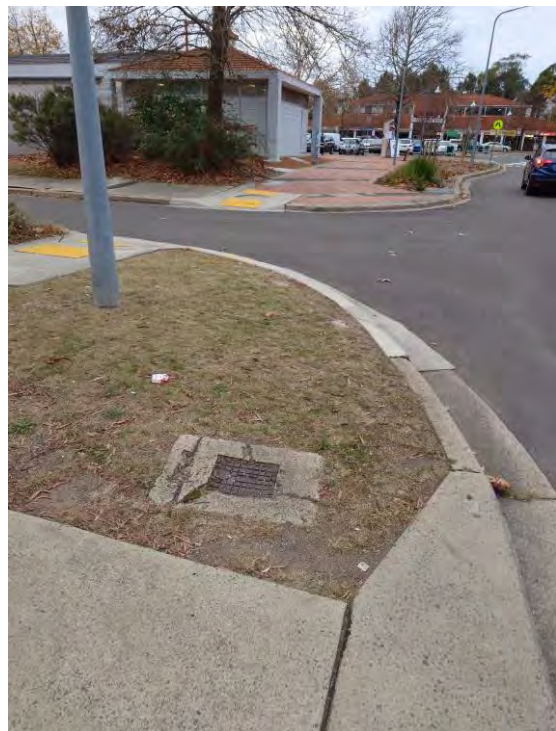
Figure 36 – Fire Hydrant in Charnwood Place (east)
