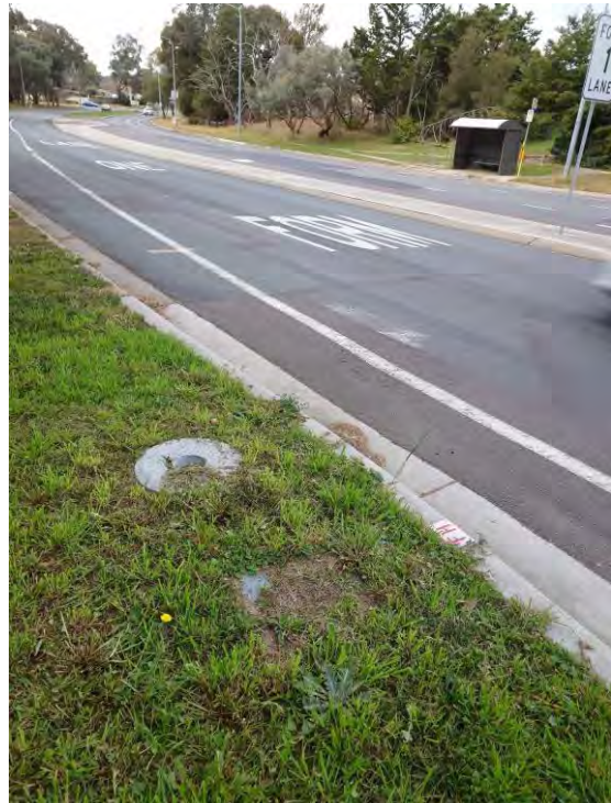
Figure 35 – Existing Fire Hydrant and Stop Valve on DN375 Main in Tillyard Drive
