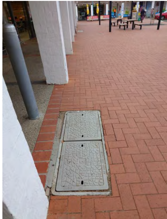
Figure 73 – Telstra Pits in South West Central Car Park
