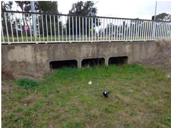
Figure 59 – Stormwater Box Culverts under Lhotsky Street
