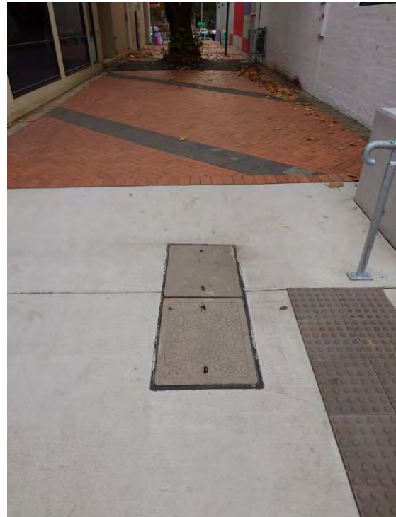
Figure 69 – Telstra Pit Between Block 3 and 47 Section 95
