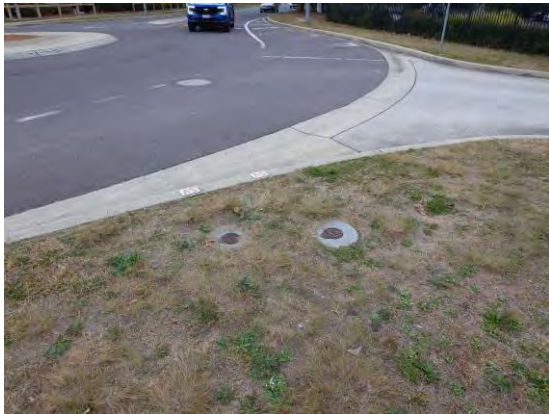
Figure 33 – Existing Stop Valves at Intersection of Lhotsky Street and Charnwood Place (east)
