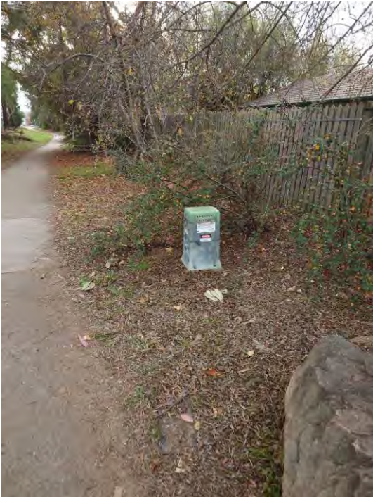
Figure 90 – Electrical Minipillar in Block 213 Section 96 North of Site
