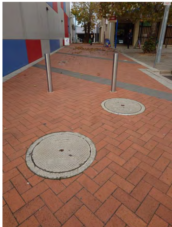
Figure 18 – Sewer Manholes over DN150 Mains Servicing Block 7 and 47 Section 95
