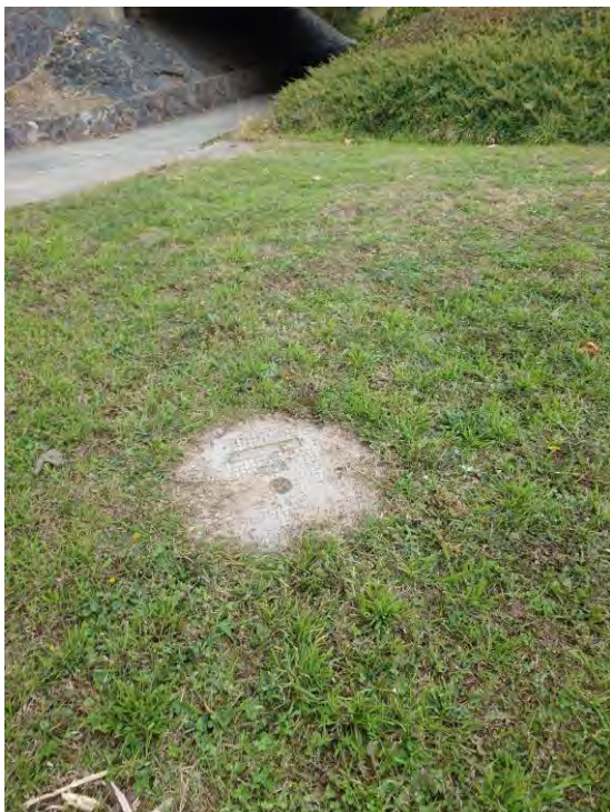
Figure 20 – Sewer Manhole over DN300 Main in Open Space (Block 11 Section 95)
