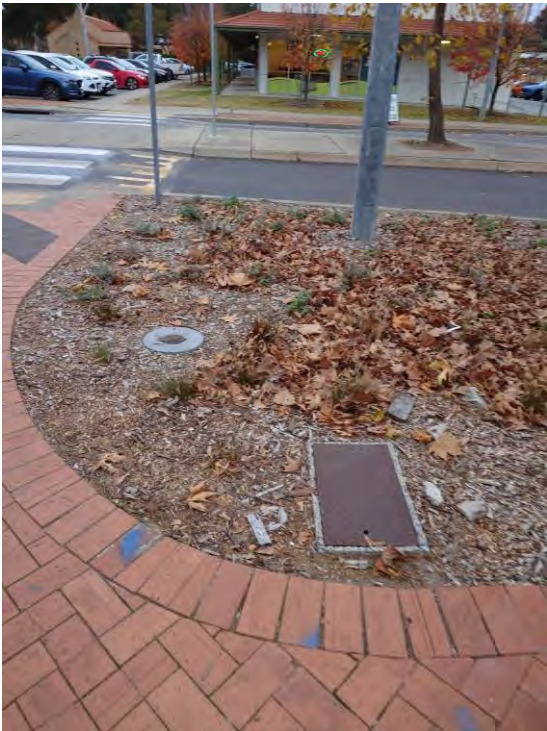
Figure 37 – Water Meter Pit and Stop Valve in Charnwood Place (east)
