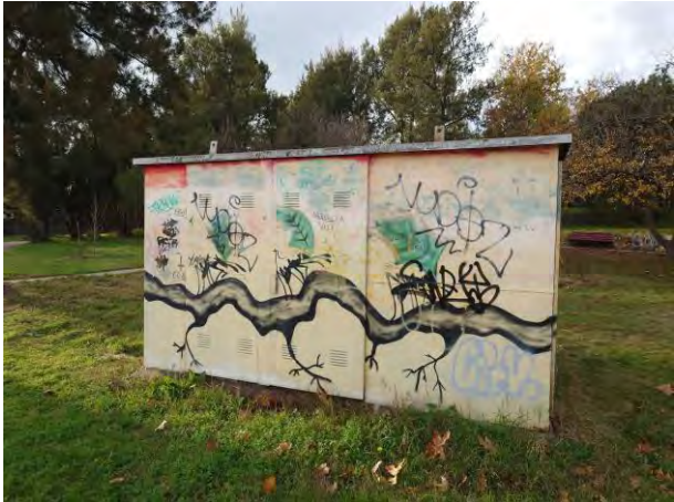
Figure 92 – Electrical Substation S 2720 North of Block 5 Section 95
