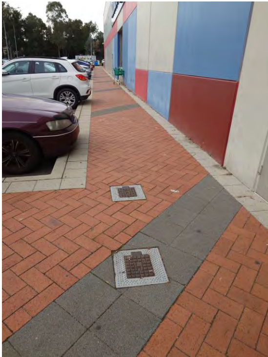
Figure 29 – Double Hydrants in Charnwood Place (west)
