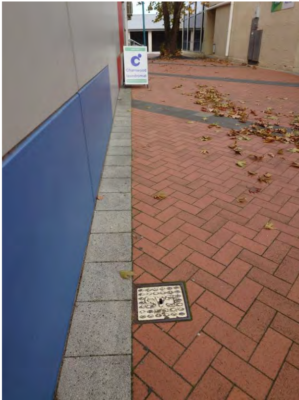
Figure 79 – Gas Isolation Valve Between Block 3 and Block 47 Section 95
