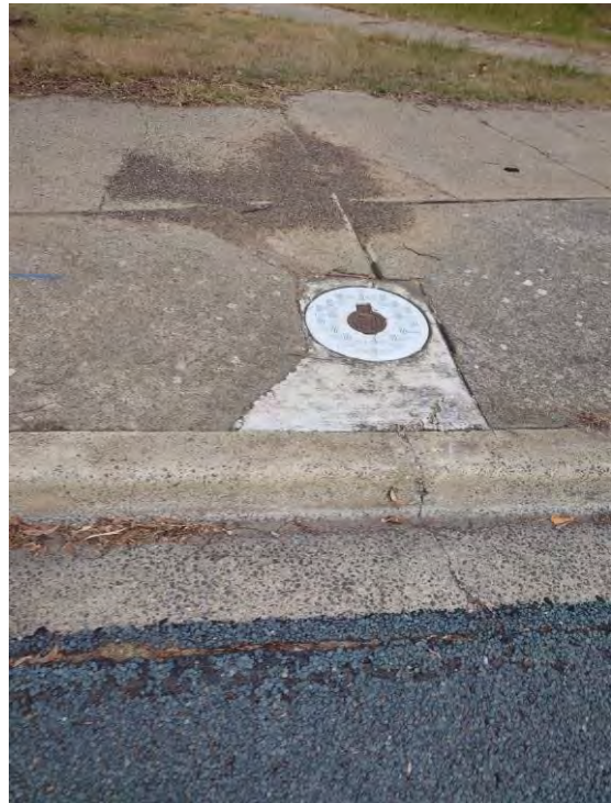
Figure 31 – Stop Valve Near Intersection of Charnwood Place (west) and Lhotsky Street
