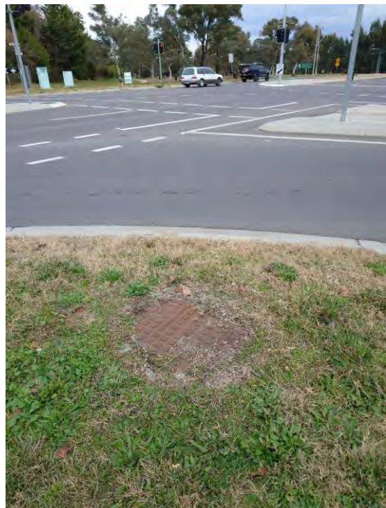
Figure 22 – Sewer Manhole over DN300 Main at Intersection of Lhotsky Street and Tillyard Drive
