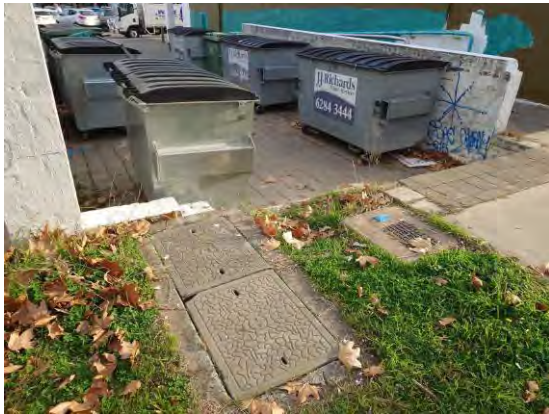
Figure 67 – Telstra Pit in Charnwood Place (west)
