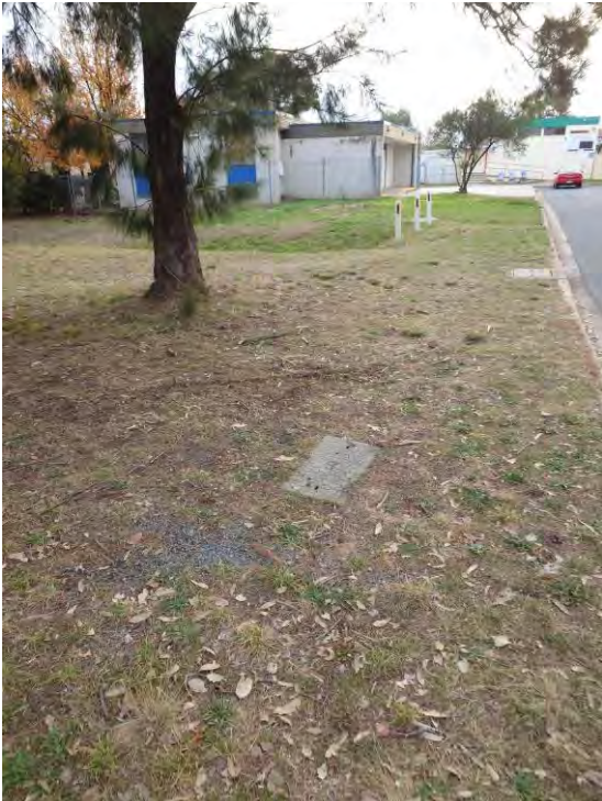
Figure 64 – Telstra Pit in Verge Place
