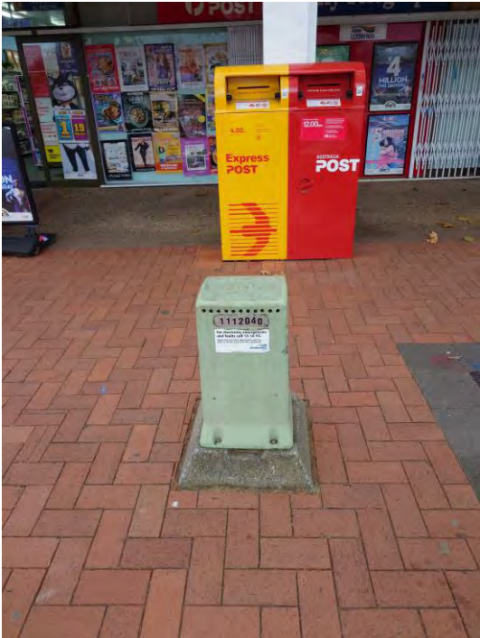
Figure 91 – Electrical Minipillar in North Central Group Centre
