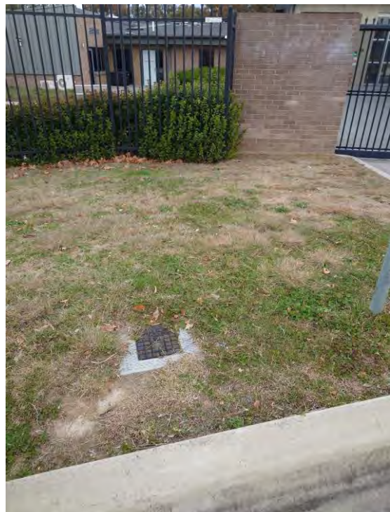
Figure 32 – Fire Hydrant on DN300 Main in Lhotsky Street
