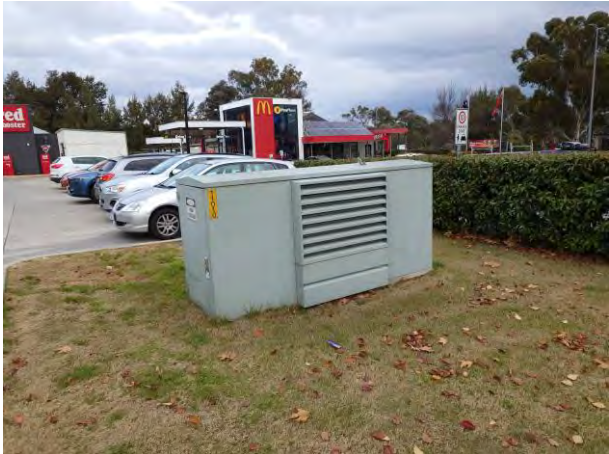
Figure 93 – Electrical Substation S 11010 in Block 44 Section 95
