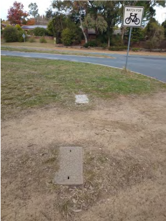
Figure 63 – Telstra Pit at Intersection of Tillyard Drive and Verge Place
