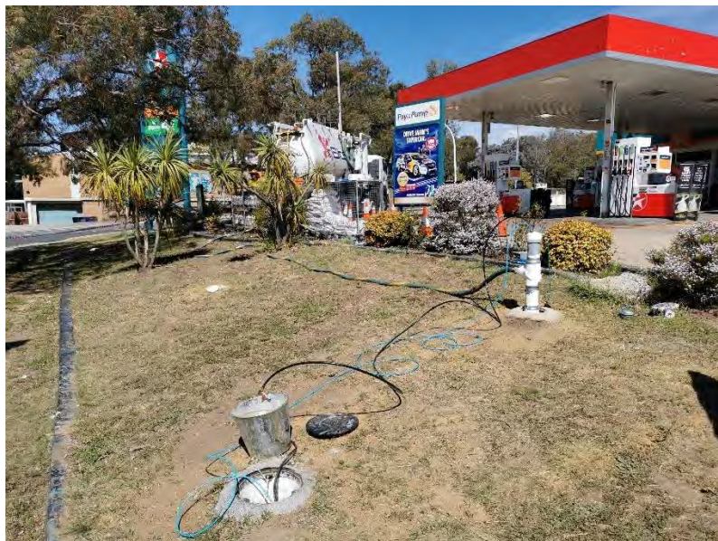
Figure 4 SVE + pumping trial showing the vacuum hose and pneumatic pump tubes connected to the extraction well head.
