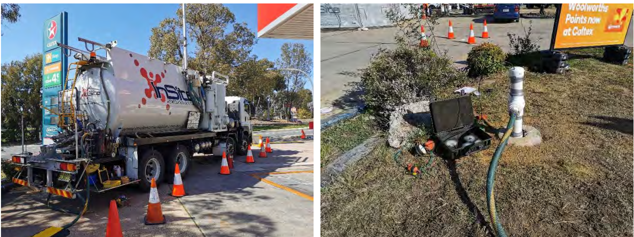
Figure 1 Truck mounted vacuum separation system (left) and extraction well head setup for SVE trial (right).
