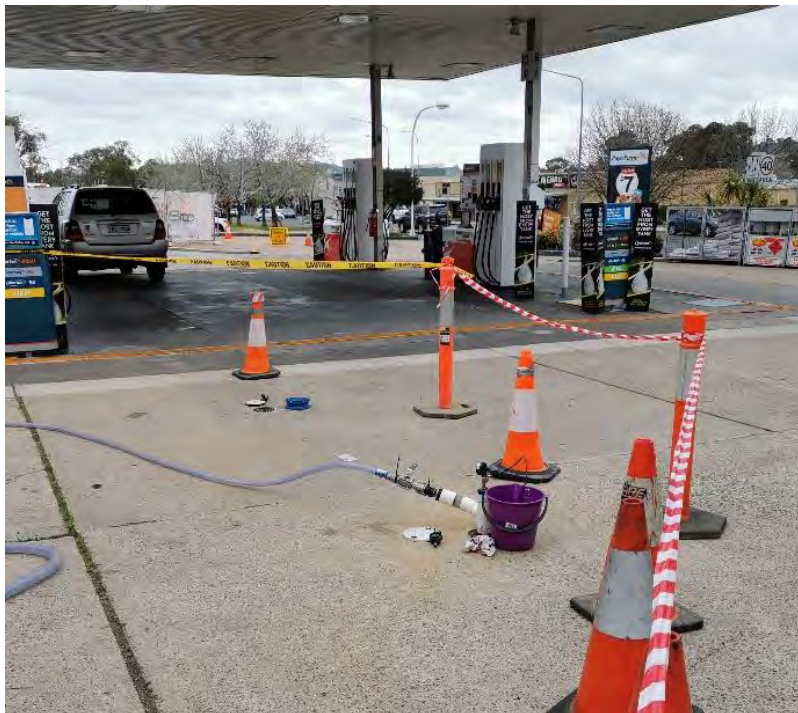
Figure 12 Chemical injection point at well head IW02
