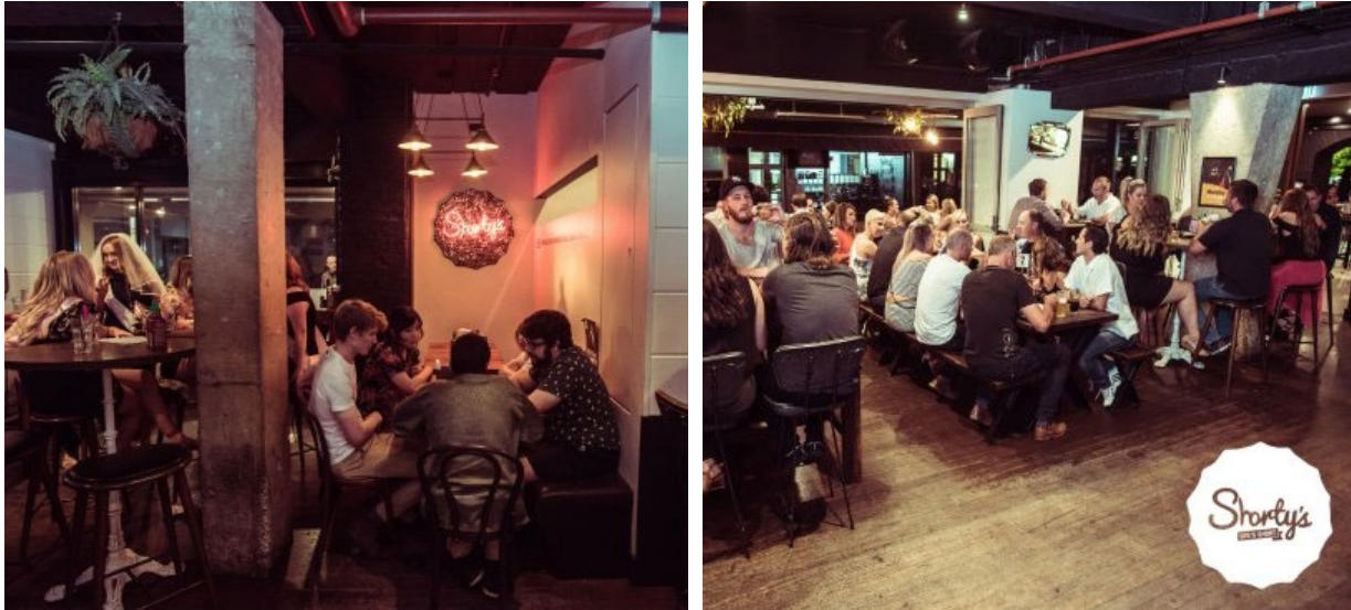
Image 14 (left), Image 15 (right). Ground floor interior (Shorty's Bar) with exposed Vierendeel Trusses (Shorty's 2018)
