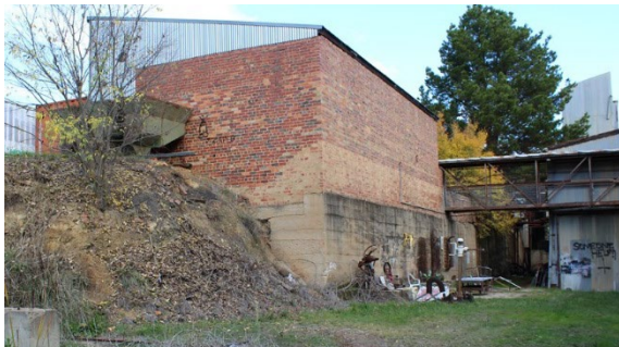
Figure 3.34 Concrete retaining wall (Element 24), showing later masonry wall constructed on top. (Source: GML, 2017)
