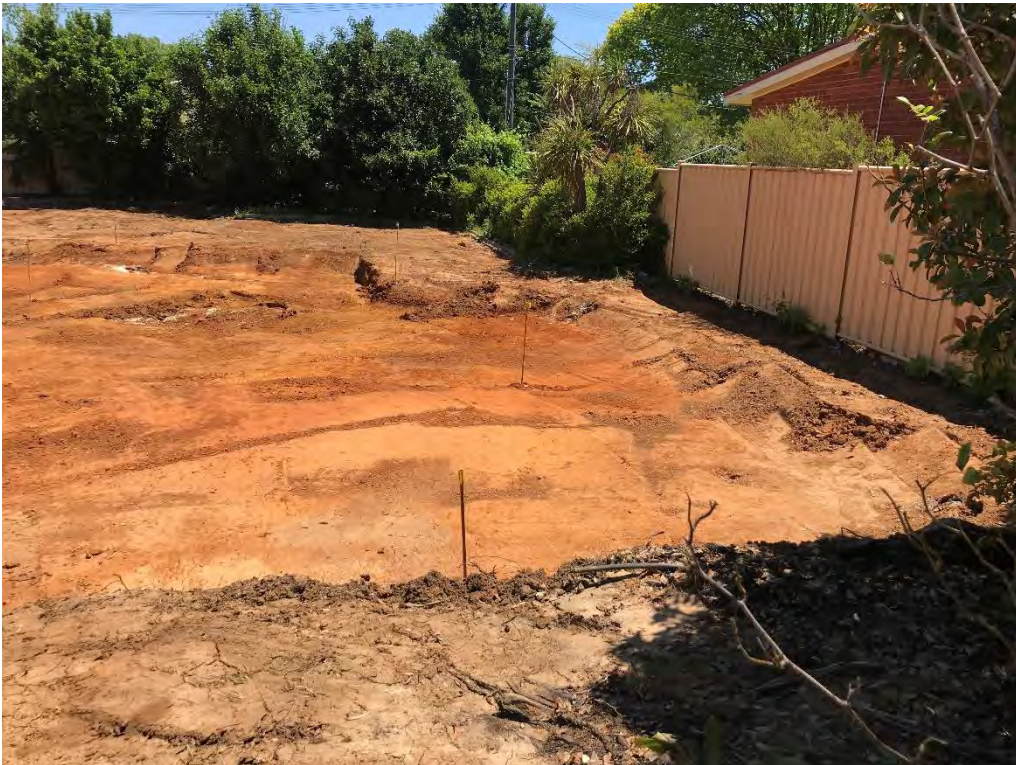
Figure 6 Soil validation sample location/s (from the left) view from the northern elevation of the housing footprint to the western boundary/demolition corner: S06, S05, S12, S11, S10 and S09.
