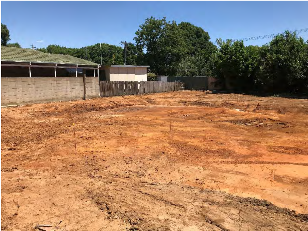
Figure 5 Soil validation sample location/s (from the left) view from the northern elevation of the housing footprint to the southern boundary/demolition corner: S08, S01, S02, S07, S03, S06 and S05.
