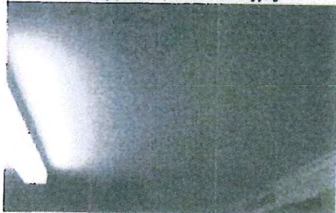
9. Garage, view of plaster sheets sagging
