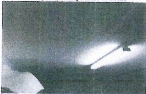
8. Garage, view of plaster sheets sagging
