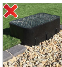
Incorrect box level
