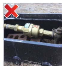
Incorrect meter height
