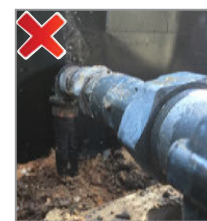
No copper risers
