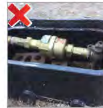
Incorrect meter height
