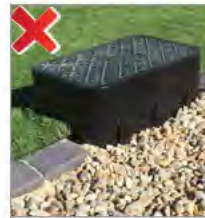
Incorrect box level
