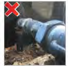
No copper risers
