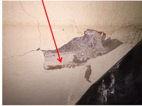
Photograph 18: Level 2, kitchenette, asbestos containing lagging to hot water pipes in wall.
