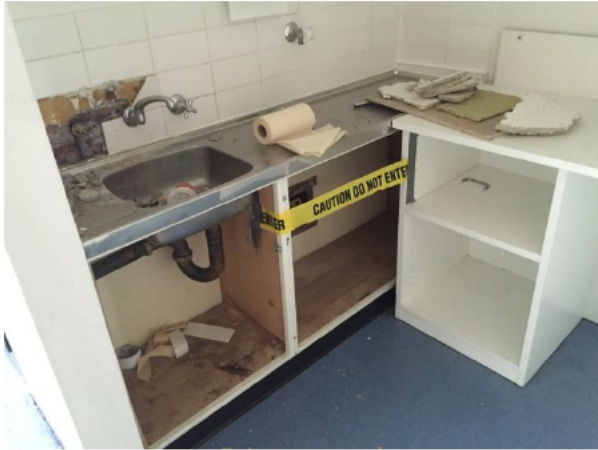
Photograph 17: Level 2, kitchenette, asbestos containing lagging to hot water pipes in wall.
