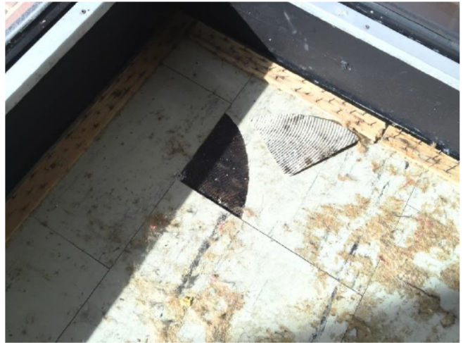
Photograph 14: Level 2, throughout entire level, asbestos cement vinyl floor tiles and blackjack adhesive beneath carpeted areas.
