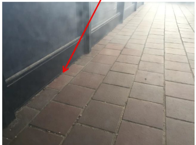
Photograph 16: Level 2, exterior balcony, asbestos containing putty used as sealant / caulking to base of window panels.
