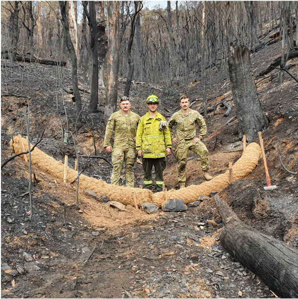
The ACT Parks and Conservation Service and the Australian Defence Force worked to install coir logs in the Upper Cotter catchment following the Orroral Valley Fire — February 2020
