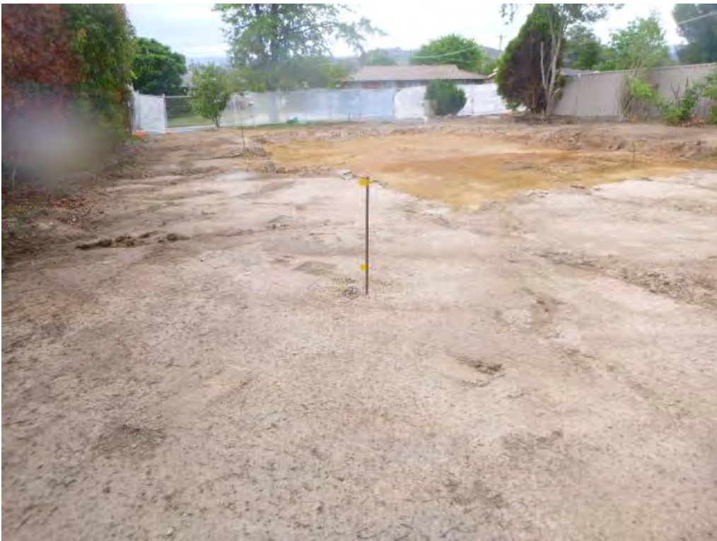
Figure 6 Soil validation sample location/s (from the left) view from the north-eastern corner of the demolition area to the southern boundary/demolition corner: S12, S10, S11, S02, S09, S06, S01, S04 and S05.
