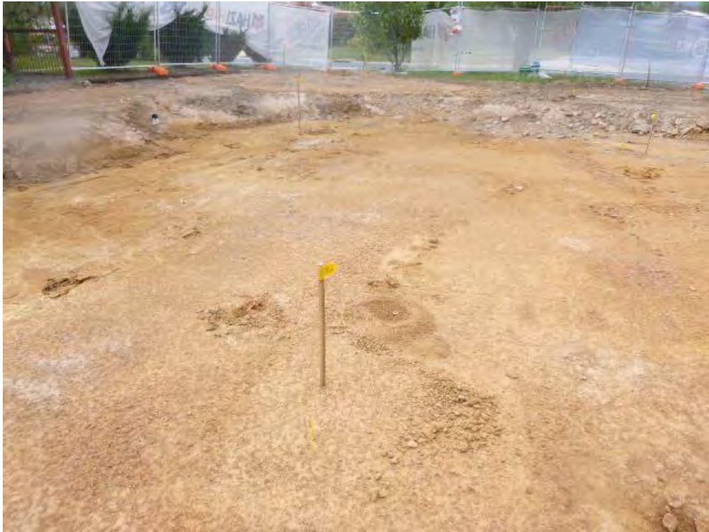
Figure 5 Soil validation sample location/s (from the left) view from the southern centre of the housing footprint to the southern boundary: S12, S11, S06, S02 and S03.
