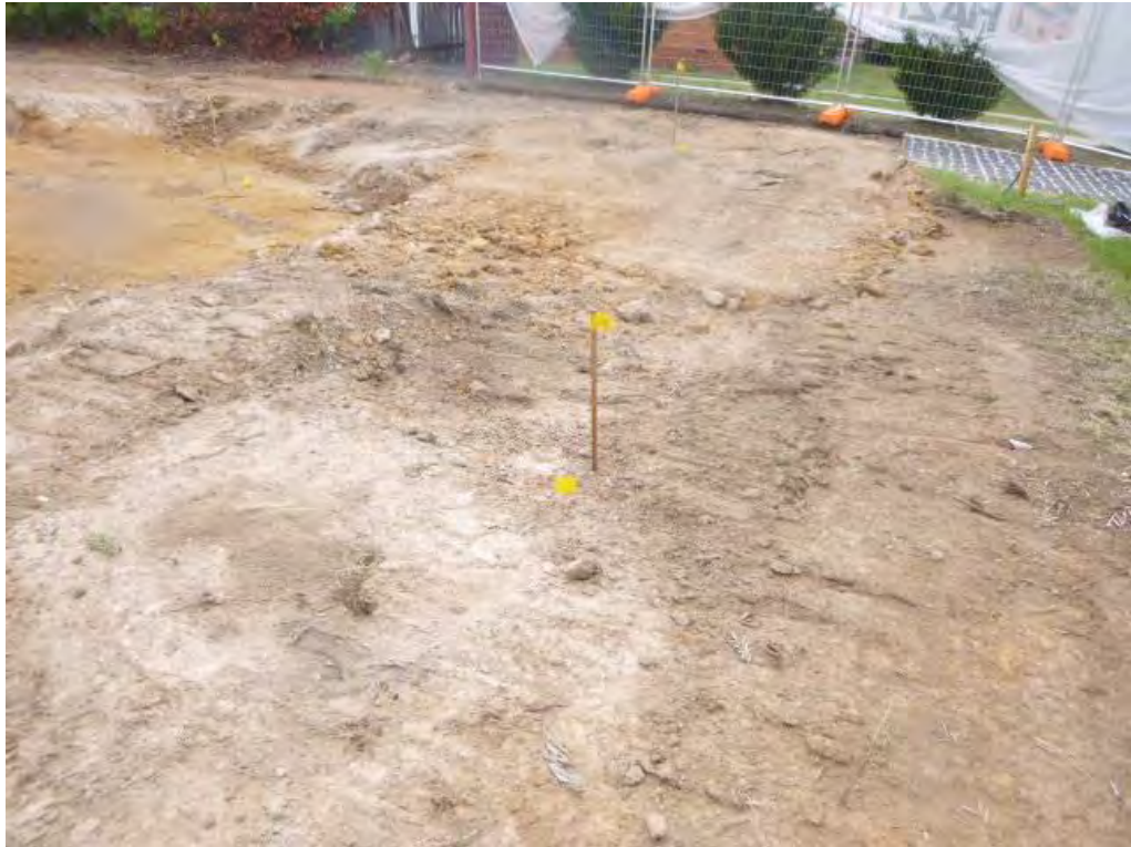
Figure 3 Soil validation sample location/s (from the left) view from the southern elevation of the demolition area to the eastern boundary: S11, S02 and S12.
