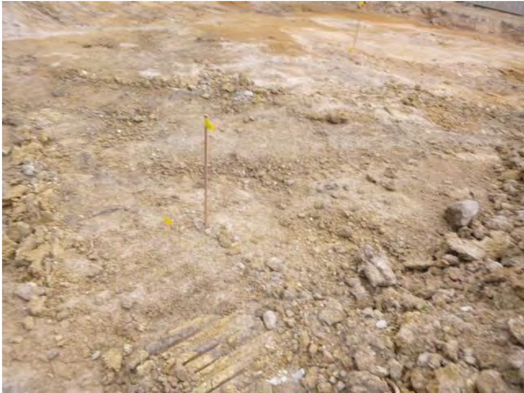
Figure 7 Soil validation sample location/s (from the left) view from the south-western corner of the demolition area to the eastern boundary: S11 and S12.
