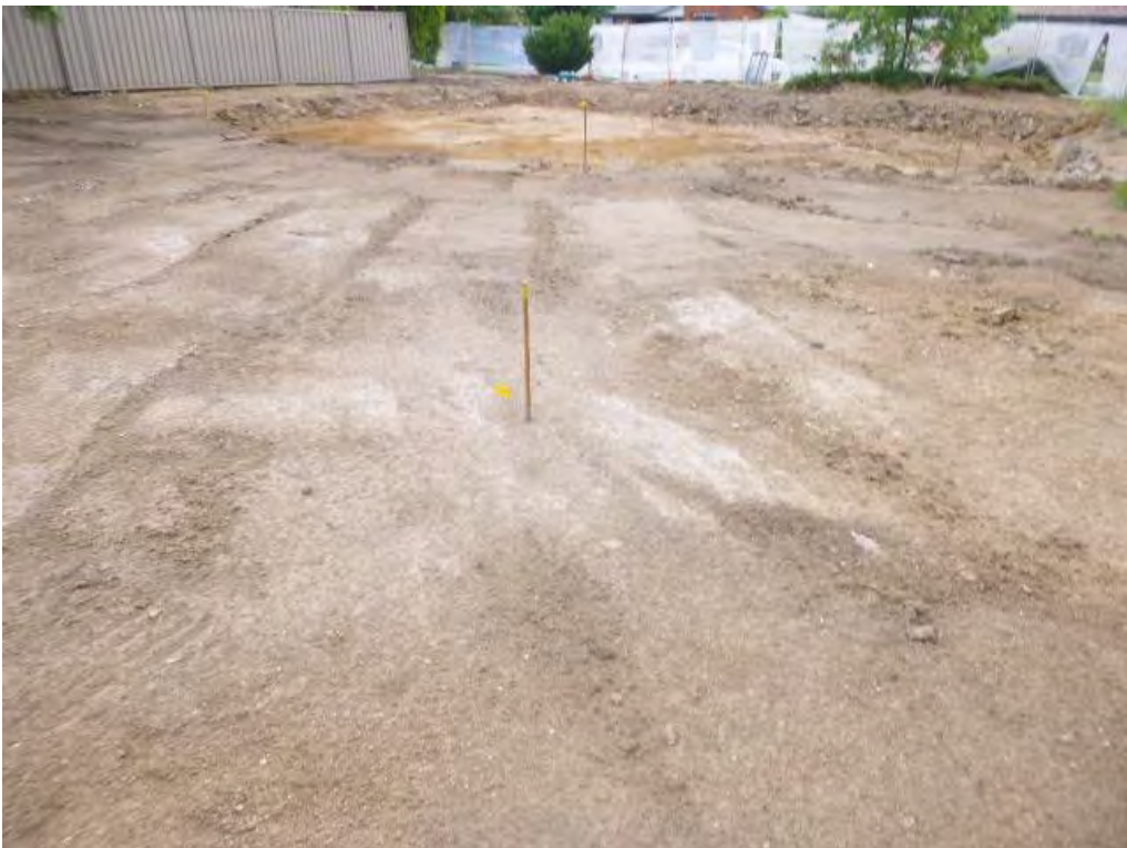
Figure 6 Soil validation sample location/s (from the left) view from the north-western corner of the demolition area to the south-eastern boundary/demolition corner: S05, S06, S03, S04, S01, S02, S09, S12 and S11.
