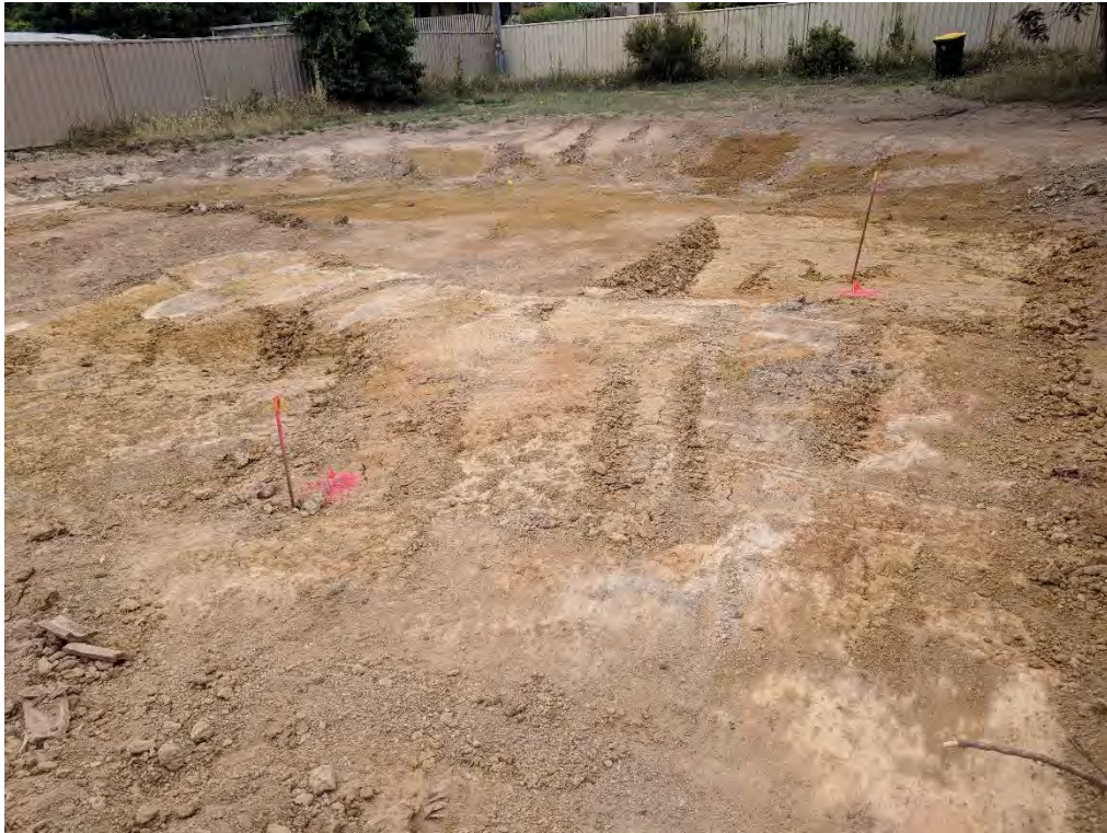
Figure 11 Final Hot Spot Soil validation sample location/s (view from the left) view from the south-eastern corner of the demolition area to the northern boundary: H/S2-7508-S01 and H/S2-7508-S04.
