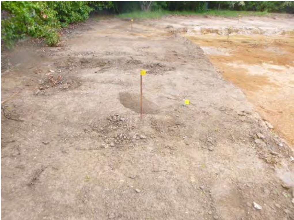
Figure 4 Soil validation sample location/s (from the left) view from the western elevation of the demolition area to the northern boundary: S04, S05, S06, S07 and S09.
