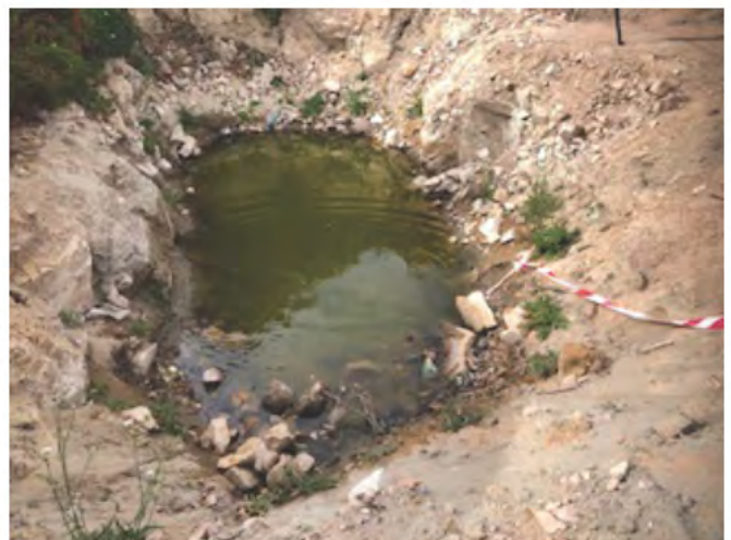
Pool excavation with water ingress
