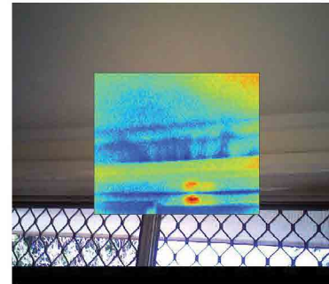
f Leakage between architrave and wall, case study 4
