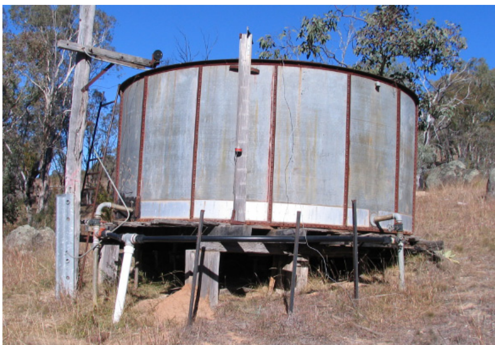
Photograph No. 14 – [REDACTED] Water Storage Tank.
