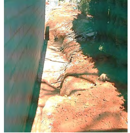
Figure 4. The excavation for the retaining wall adjacent to the trees that are shown in Figure 3. Photograph by Alan Mann 31 August 2006.
