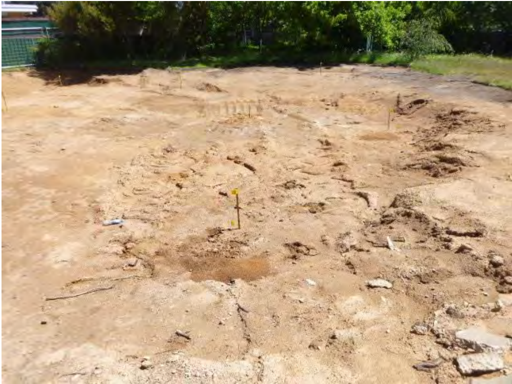
Figure 3 Soil validation sample location/s (from the left) view from the south-eastern corner of the demolition area to the western boundary/demolition corner: S09, S07, S06, S01, S04, S05 and S03.
