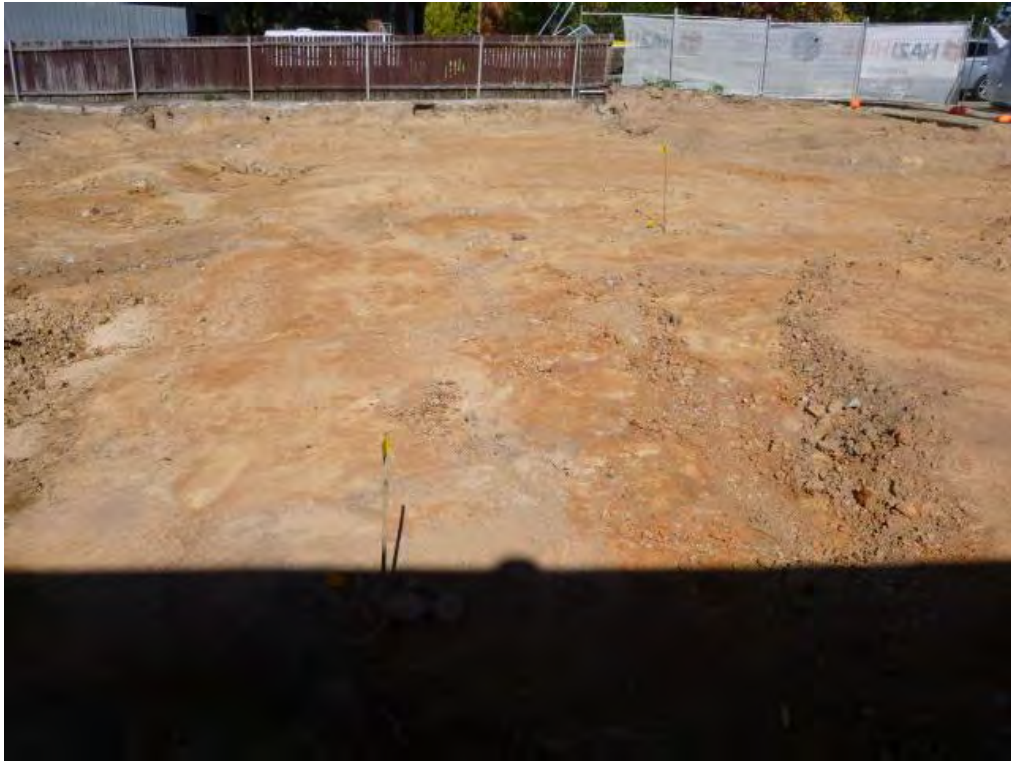
Figure 5 Soil validation sample location/s (from the left) view from the northern elevation of the demolition zone to the southern boundary: S-07, S-04, S-06 and S-05.
