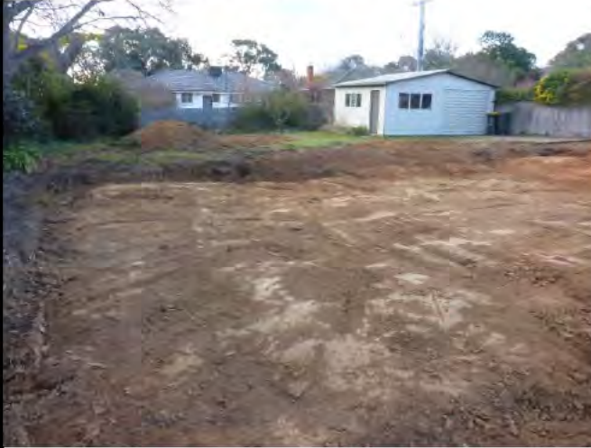
Photograph 1: 27 Rivett Street, Hackett view to north showing excavated area with retained garage to the rear of the site.
