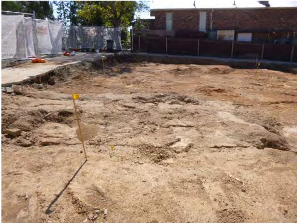
Figure 3 Soil validation sample location/s (from the left) view from the south-eastern boundary corner to the northern boundary: S-01, S-02, S-03, S-05 and S-04.
