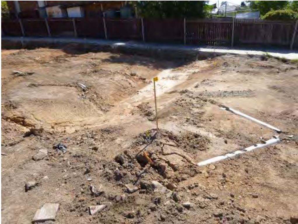
Figure 7 Soil validation sample location/s (from the left) view from S-11 to the northern boundary: S-04, S-09, S-11 and S-12.
