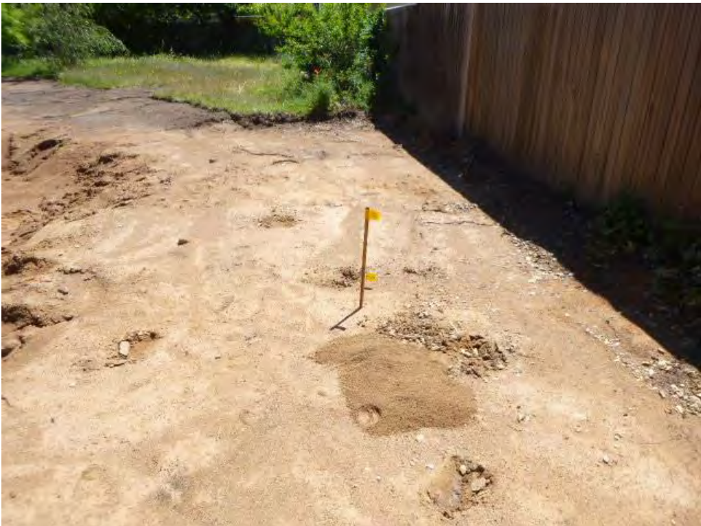
Figure 4 Soil validation sample location/s (from the left) view from the south-eastern corner of the demolition area to the eastern boundary: S02.
