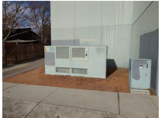
Figure 69 – Electrical Substation S 9144 and Distribution Box in North East Corner of Block 42 Section 50
