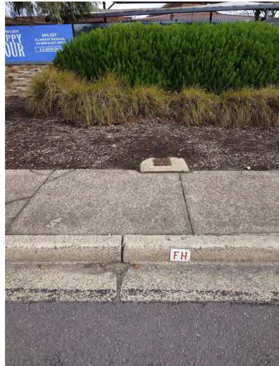
Figure 25 – Fire Hydrant in Bowman Street (west)
