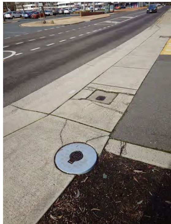
Figure 26 – Stop Valve in Bowman Street (west) for Football Club Service Tie (near)
