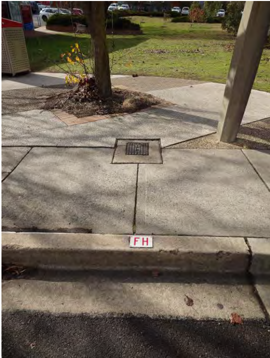
Figure 22 – Fire Hydrant on DN300 Main in Redfern Street
