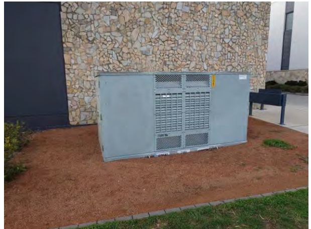
Figure 68 – Electrical Substation S 11041 South West of Site
