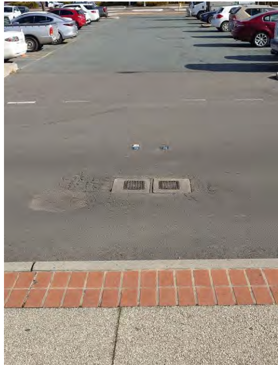
Figure 29 – Double Fire Hydrants North West of Block 42 Section 50
