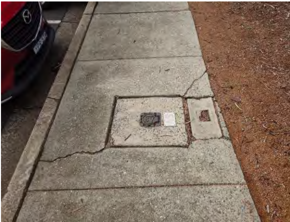
Figure 19 – Stop Valve in South East Car Park
