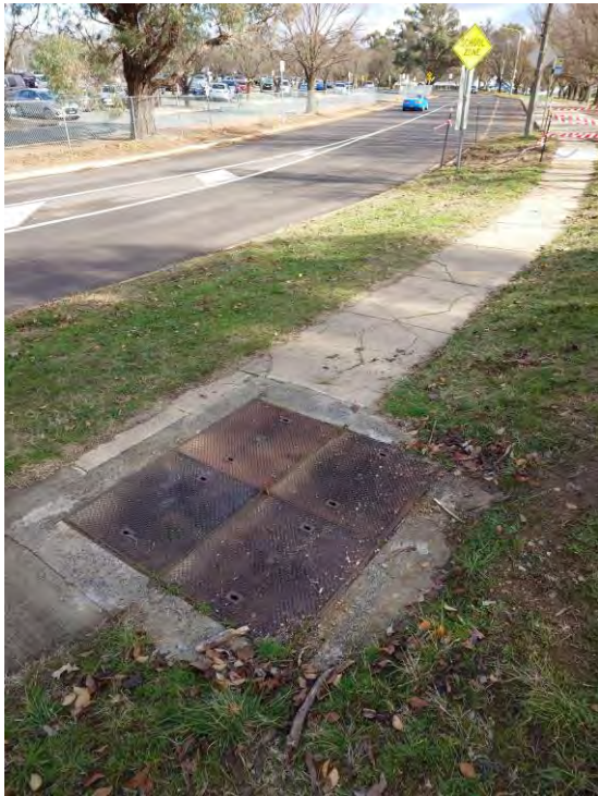
Figure 44 – Telstra Pit in Northern Verge of Bowman Street (north)
