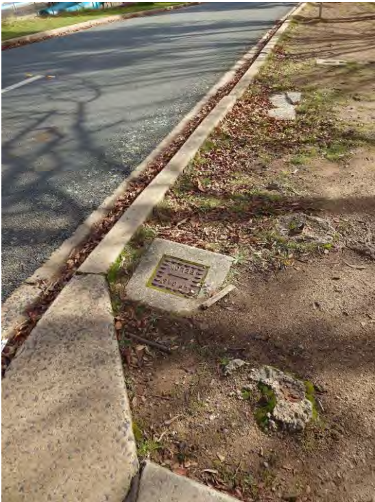
Figure 56 – Gas Marker in Halloran Close Near Intersection with Bowman Street (north)
