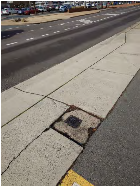
Figure 27 – Stop Valve in Bowman Street (west) for Branch into Group Centre
