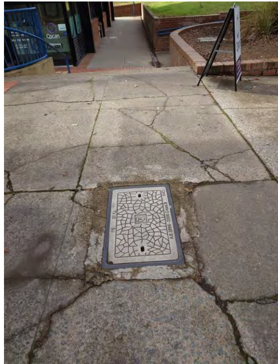
Figure 42 – Telstra Pit in Northern Area of Block 45 Section 50
