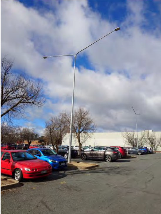
Figure 58 – TCCS Streetlight in Northern Car Park
