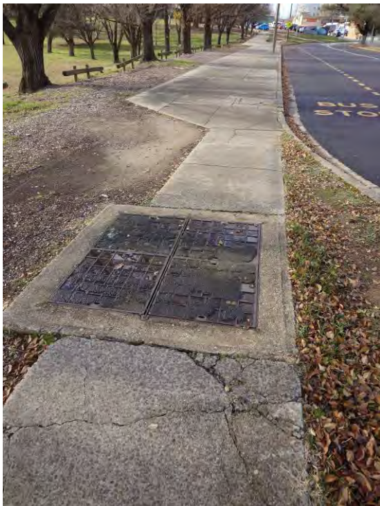
Figure 45 – Telstra Pit in Northern Verge of Bowman Street (north)
