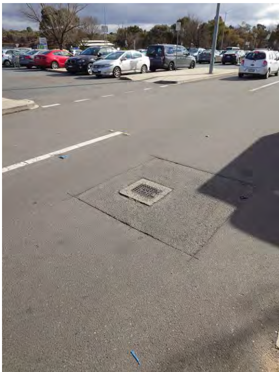
Figure 28 – Existing Fire Hydrant in West Car Park
