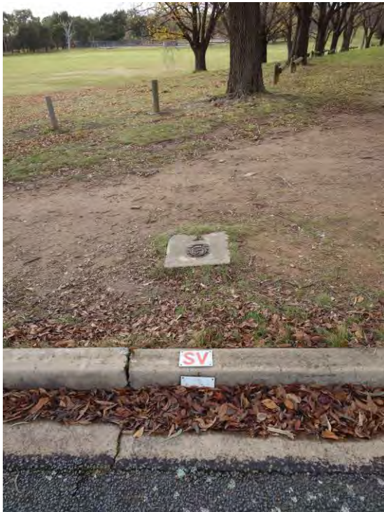
Figure 23 – Stop Valve at Intersection of Bowman Street (north) and Halloran Close
