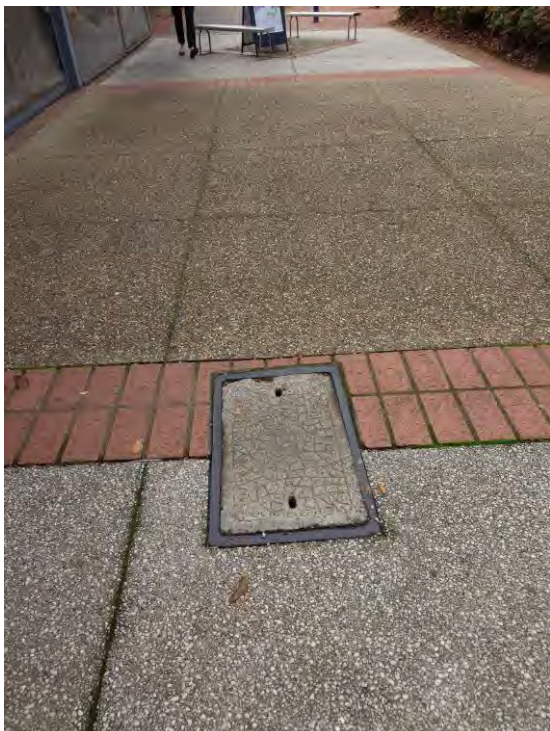
Figure 41 – Telstra Pit in Northern Verge of Jamison Centre (south) Internal Access Road
