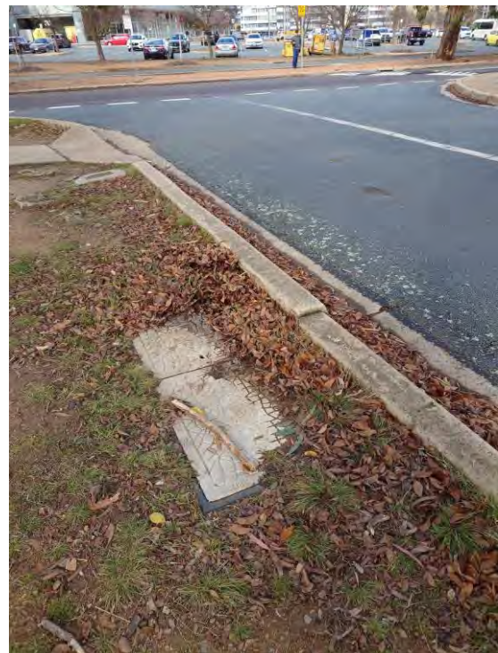
Figure 47 – Telstra Pit at the Intersection of Bowman Street (north) and Halloran Close
