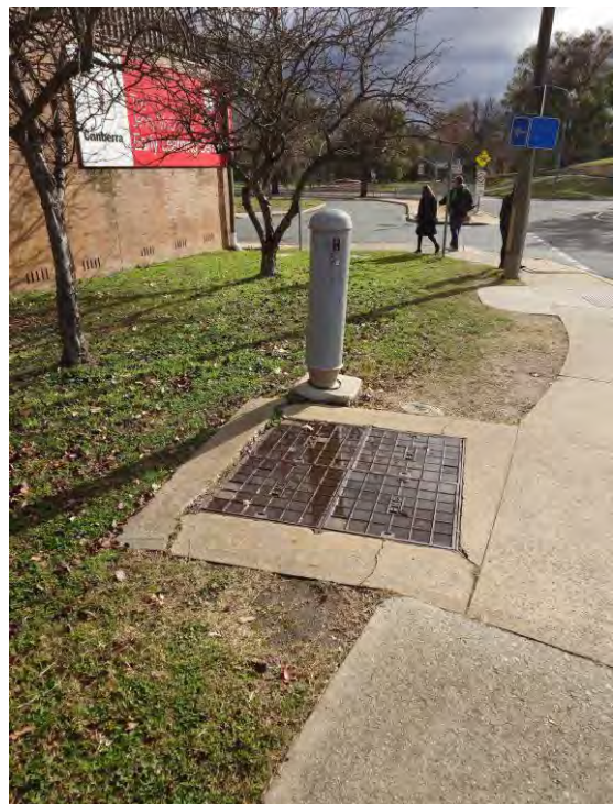
Figure 43 – Telstra Pit and Pillar Near the Intersection of Jamison Centre (east) Internal Access Road and Bowman Street (east)
