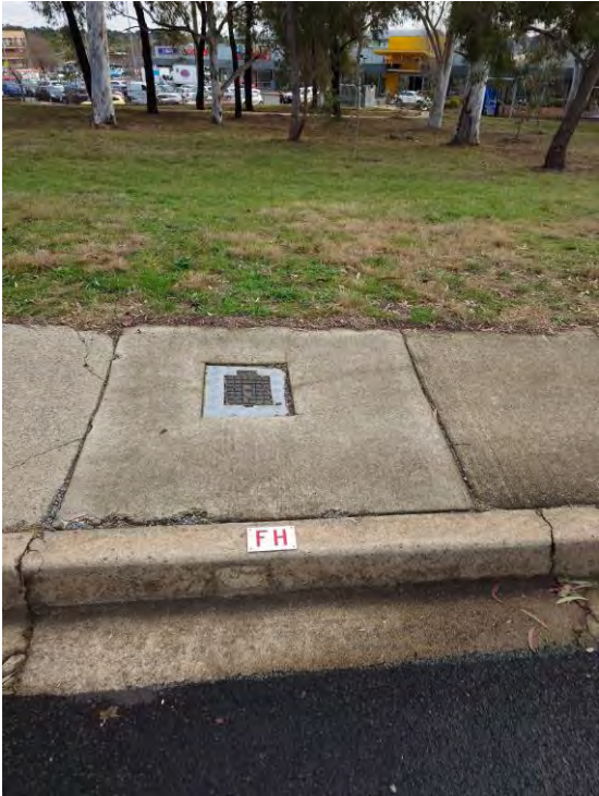
Figure 20 – Fire Hydrant on DN300 Main in Redfern Street
