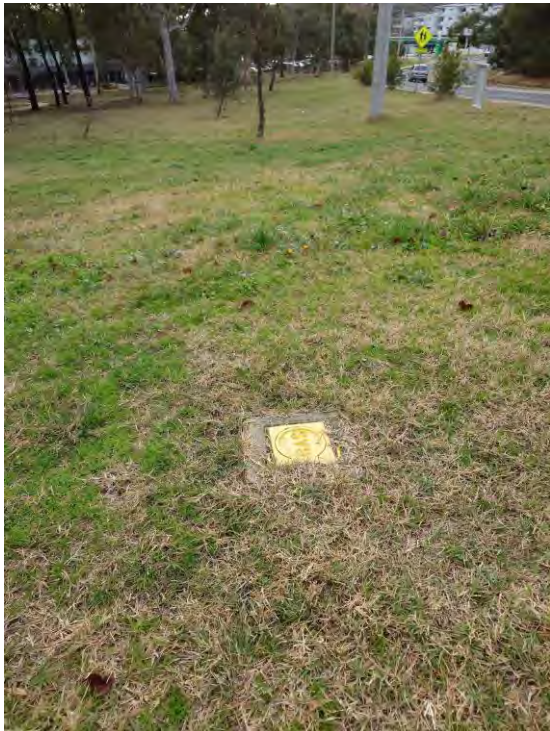
Figure 52 – Gas Isolation Valve in Northern Verge of Redfern Street
