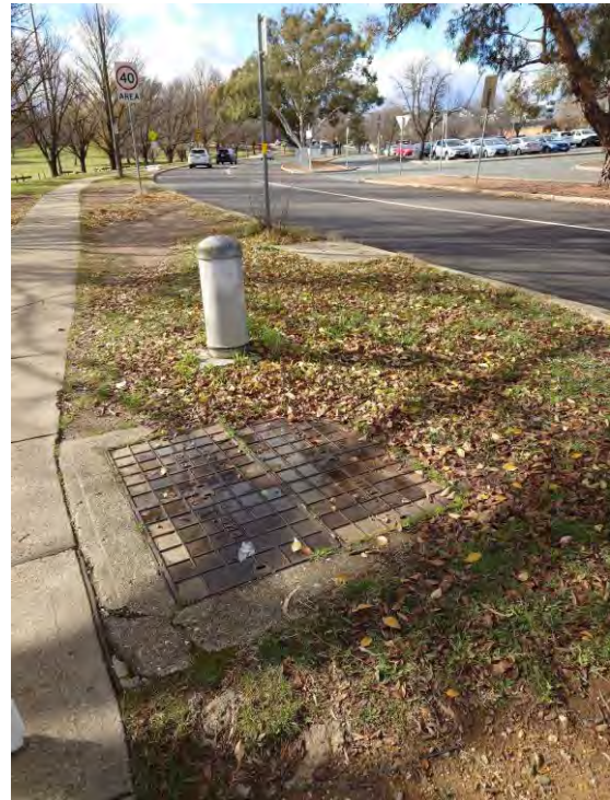
Figure 46 – Telstra Pit and Pillar Near Intersection of Bowman Street (north) and Halloran Close
