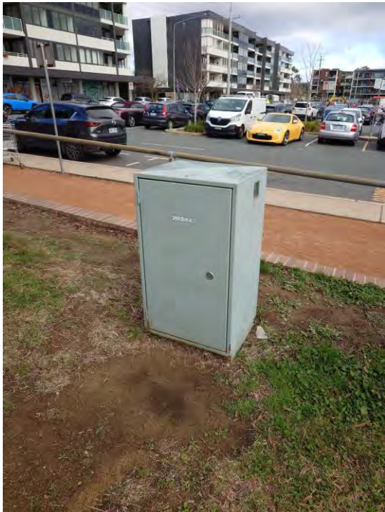
Figure 66 – Electrical Distribution Box Near Jamison Centre Internal Access Road (south)
