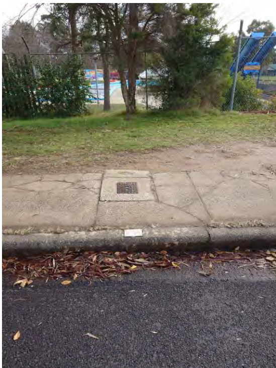
Figure 24 – Fire Hydrant in Bowman Street (north)
