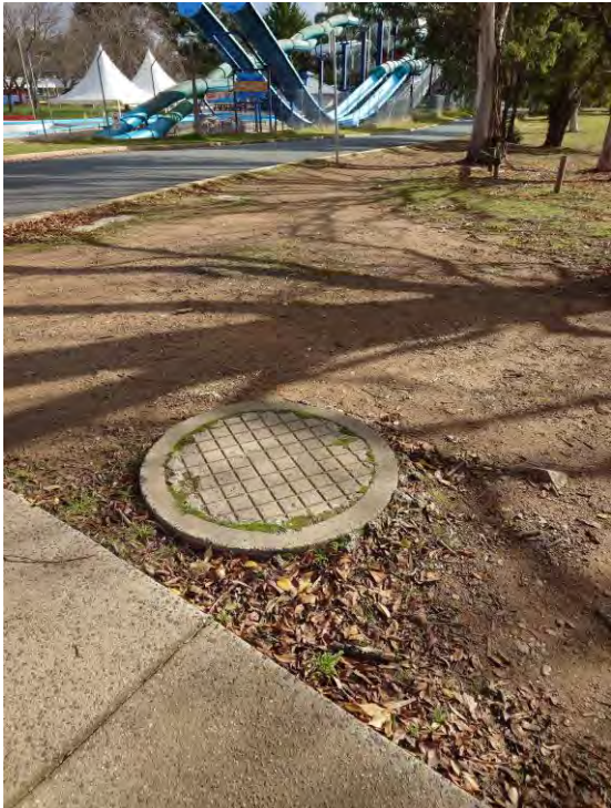
Figure 17 – Sewer Manhole over DN225 Main at Intersection of Bowman Street and Halloran Close
