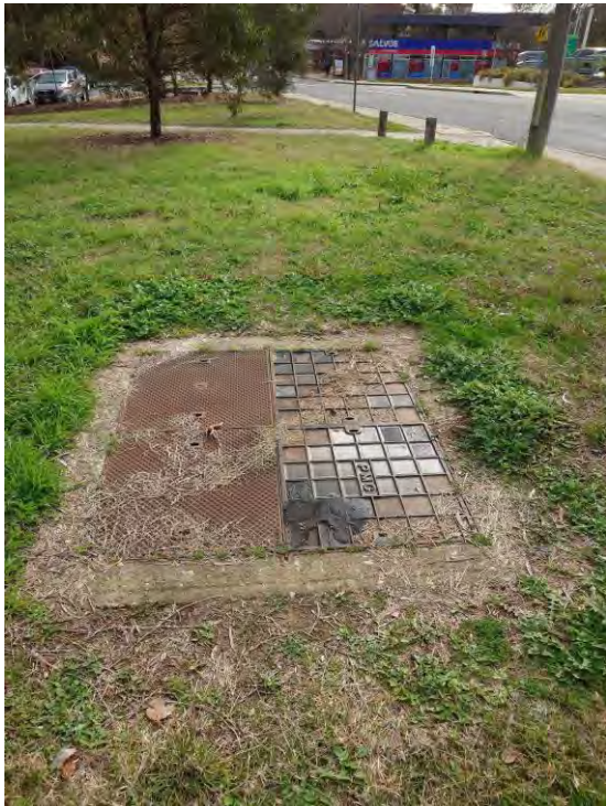
Figure 40 – Telstra Pit at the Intersection of Bowman Street (east) and Redfern Street.
