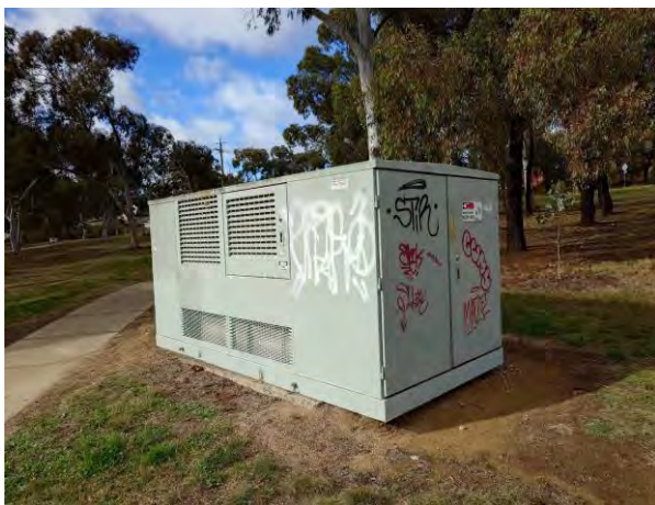
Figure 67 – Electrical Substation S 9163 Near Jamison Centre Internal Access Road (south)
