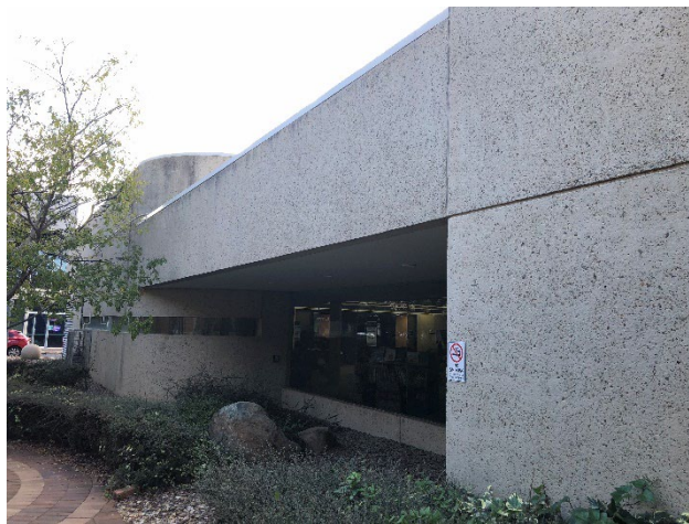
Figure 14 Recess along the southern facade for protected full height glazing, (ACT Heritage, 2020)
