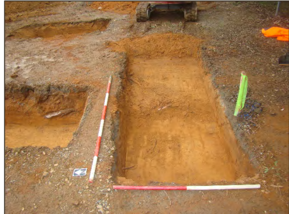
Figure 16. TT4, after excavation (2600 mm x 1100 mm x 450 mm). TT1 and TT3 are visible to the left of TT4 in the foreground and background, respectively (facing east).
