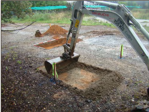
Figure 15. Mechanical excavation of the initial 50 mm spits at TT4. TT1 is visible in the background (facing north-west).
