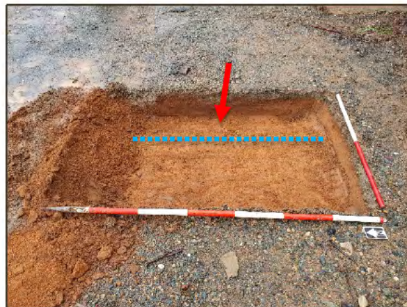
Figure 8. The base of TT1 with a service line (indicated by blue dashed line) containing yellow plastic tape running along the east end of the trench (facing east).
