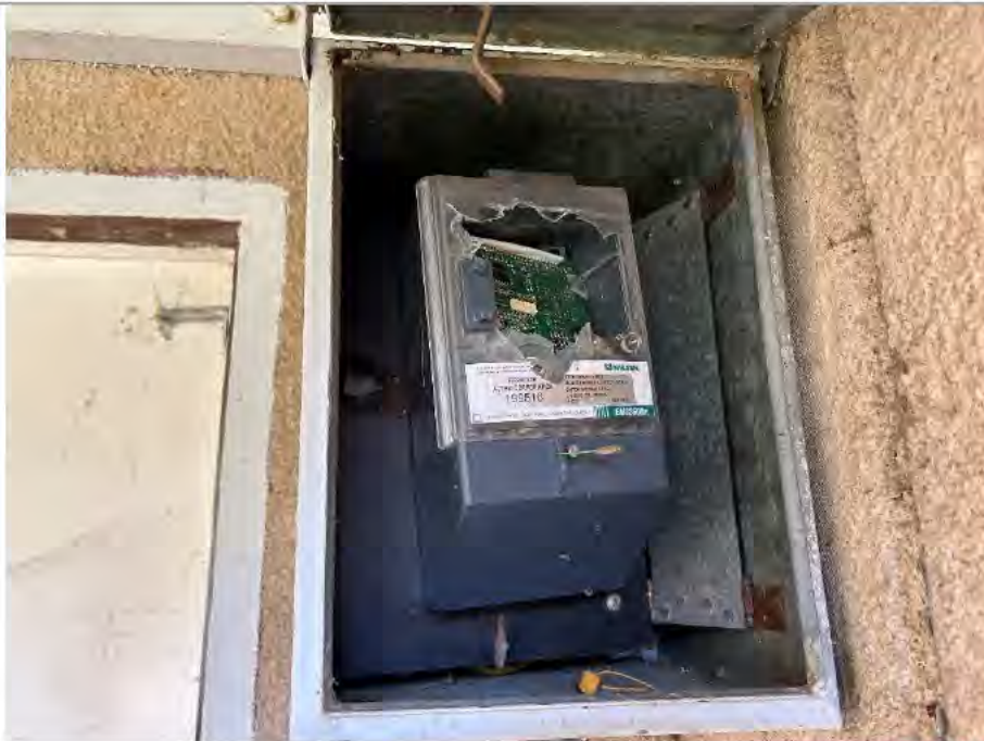
Item no. LDJ01624-2 Backing to electrical switchboard
