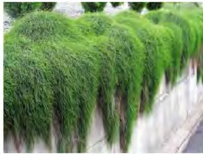
Precast concrete planter boxes
