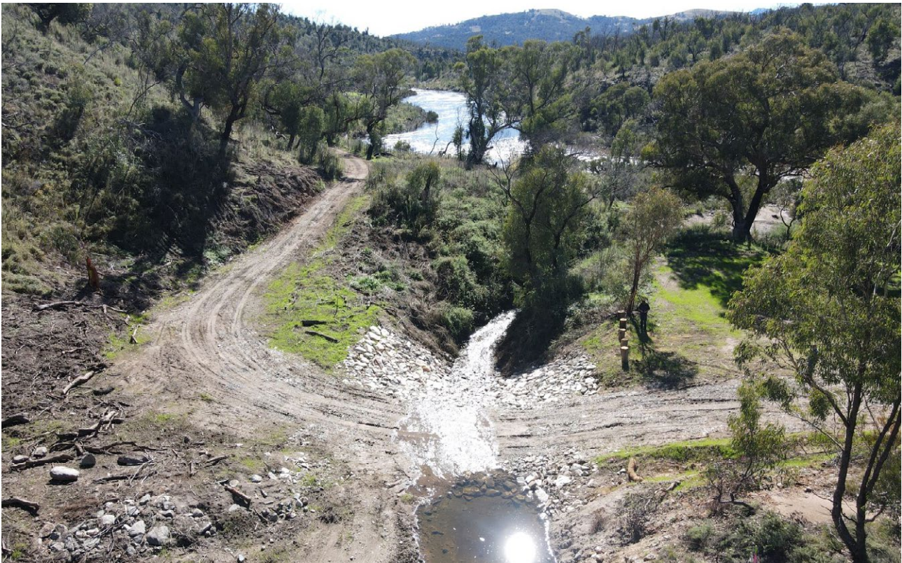
Erosion control works carried out at this site by the NSW Soil Conservation Service are part of bushfire recovery efforts to stabilise mass movement of sediment (seen upstream of rock flume) and prevent it from smothering aquatic habitat in the upper Murrumbidgee River downstream. Photo: Ashley Bolton, NSWSCS
