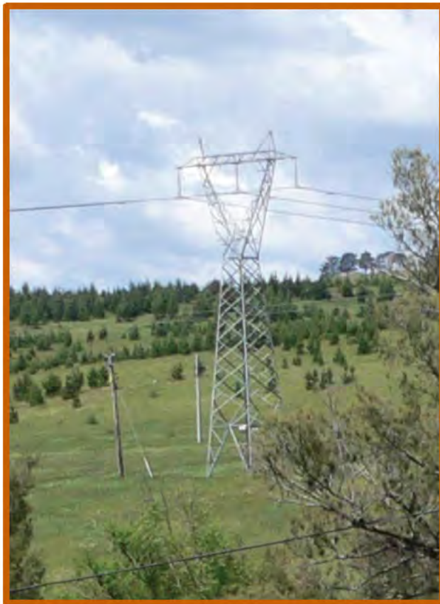
Figure 19: 132 kV Transmission Tower Adjacent to JGD
