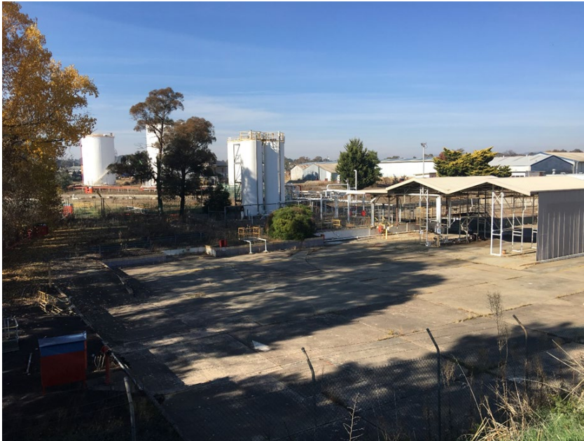
Figure 3 Residual fuel storage infrastructure onsite
