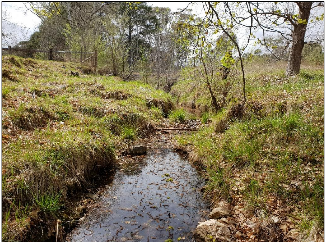
Figure 3.2 View along Halls Creek showing erosion
