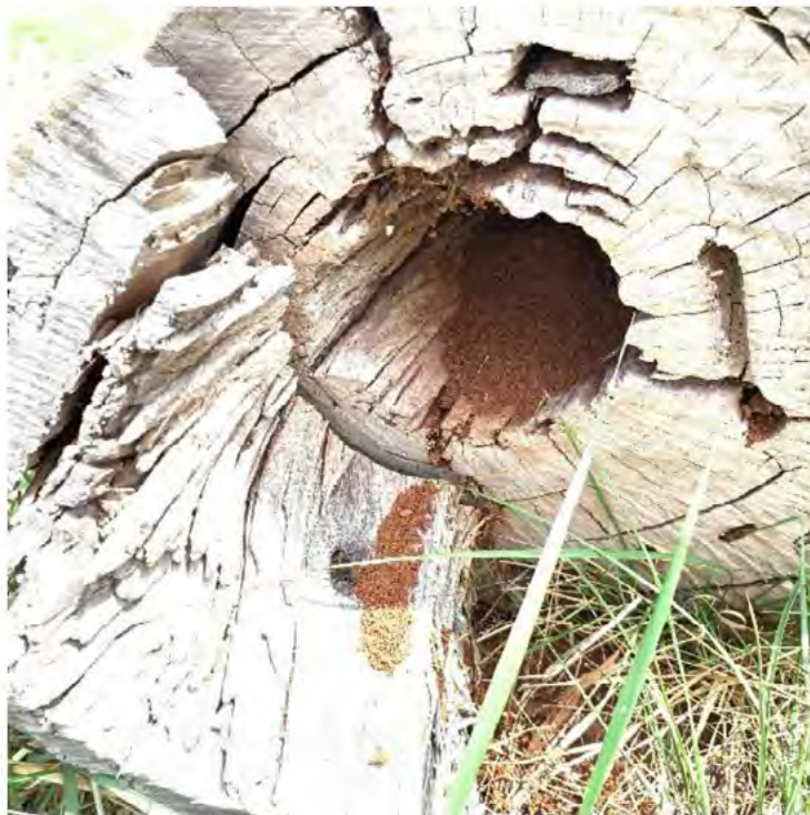
Image two: evidence of termite activity
