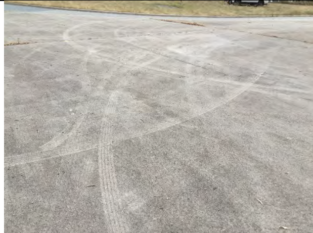
4 17Feb17 Southern Intersection Mortimer Lewis and Drakeford Drives. Vehicle tracks on concrete divider, Mortimer Lewis Drive side.
