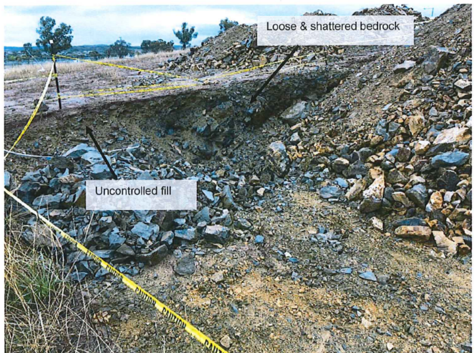
Photo 2 (right) – 26/2/2018 – View of the site cut in the western corner of the site, showing the loose, shattered bedrock extending to >2.8m depth.
