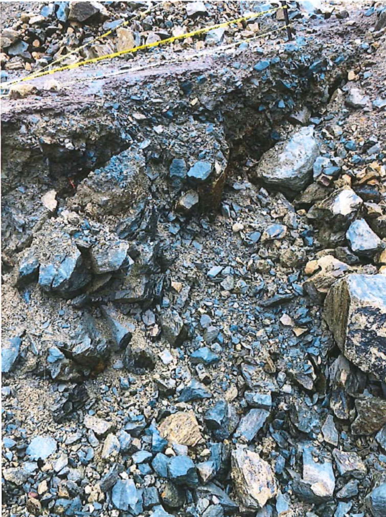
Photo 3 (above) – 26/2/2018 – Close up view of the loose & shattered bedrock.
