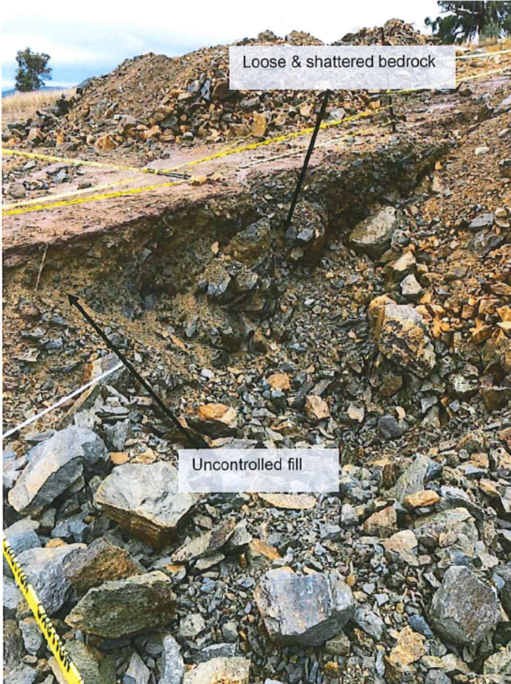
Photo 1 (left) – 26/2/2018 – View of the site cut in the western corner of the site, showing the loose, shattered bedrock extending to >2.8m depth.
