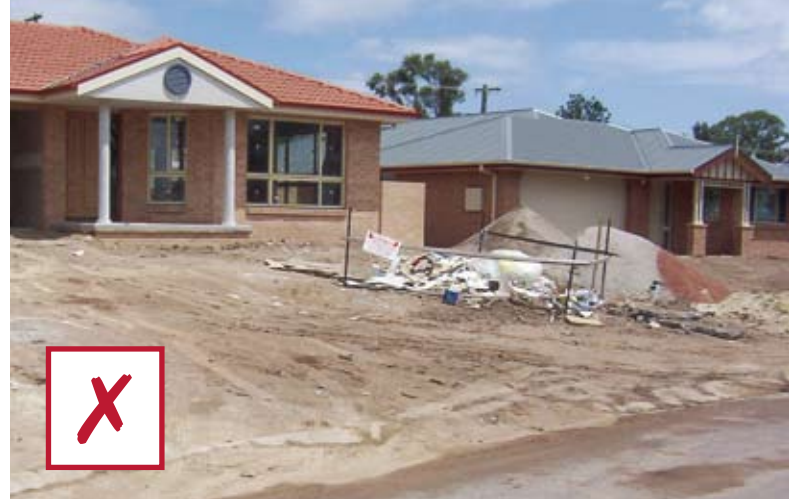
Bad building practices
